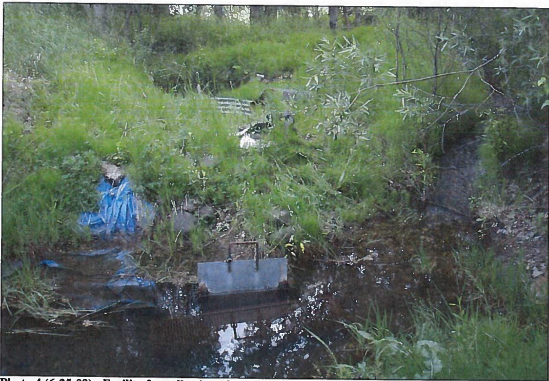
Photo 4 (6-25-09) - Facility for collection of seepage from the dam. This feature exists on the east side of the embankment. At the time, the rate of flow in the ditch (right) was estimated ~20-25 gpm.
