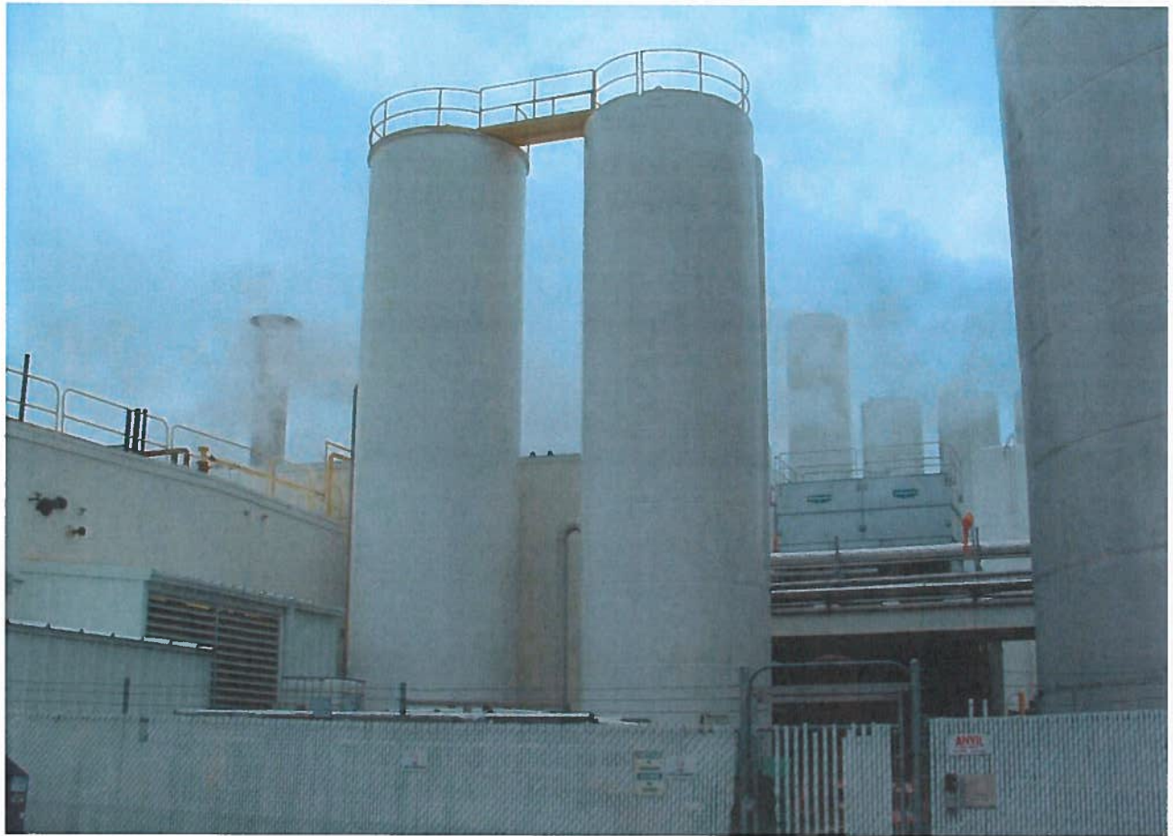
Water storage tanks – 40,000 gallon each
