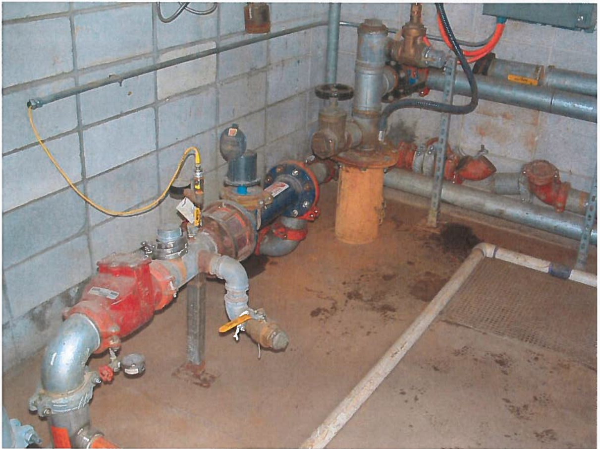
Well No. 1 – Casing and mechanical piping. 40-hp submersible pump in well.
