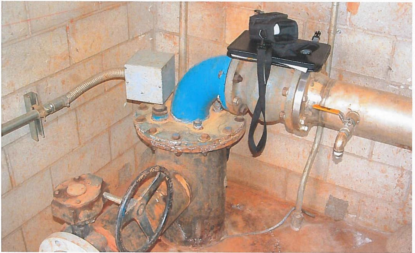
Well No. 2 – Well casing and submersible pump discharge elbow.
