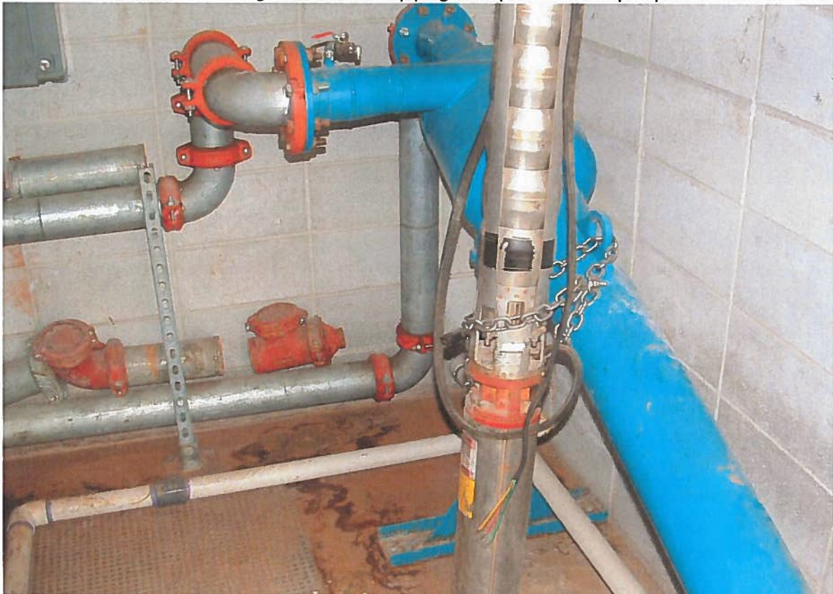
Well No. 1 – sand separator (in blue) and back-up pump (20-hp)
