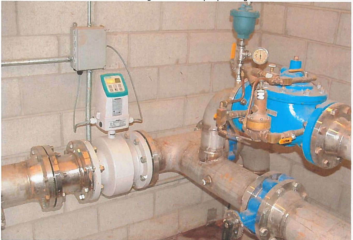
Well No. 2 mechanical piping and flow meter
