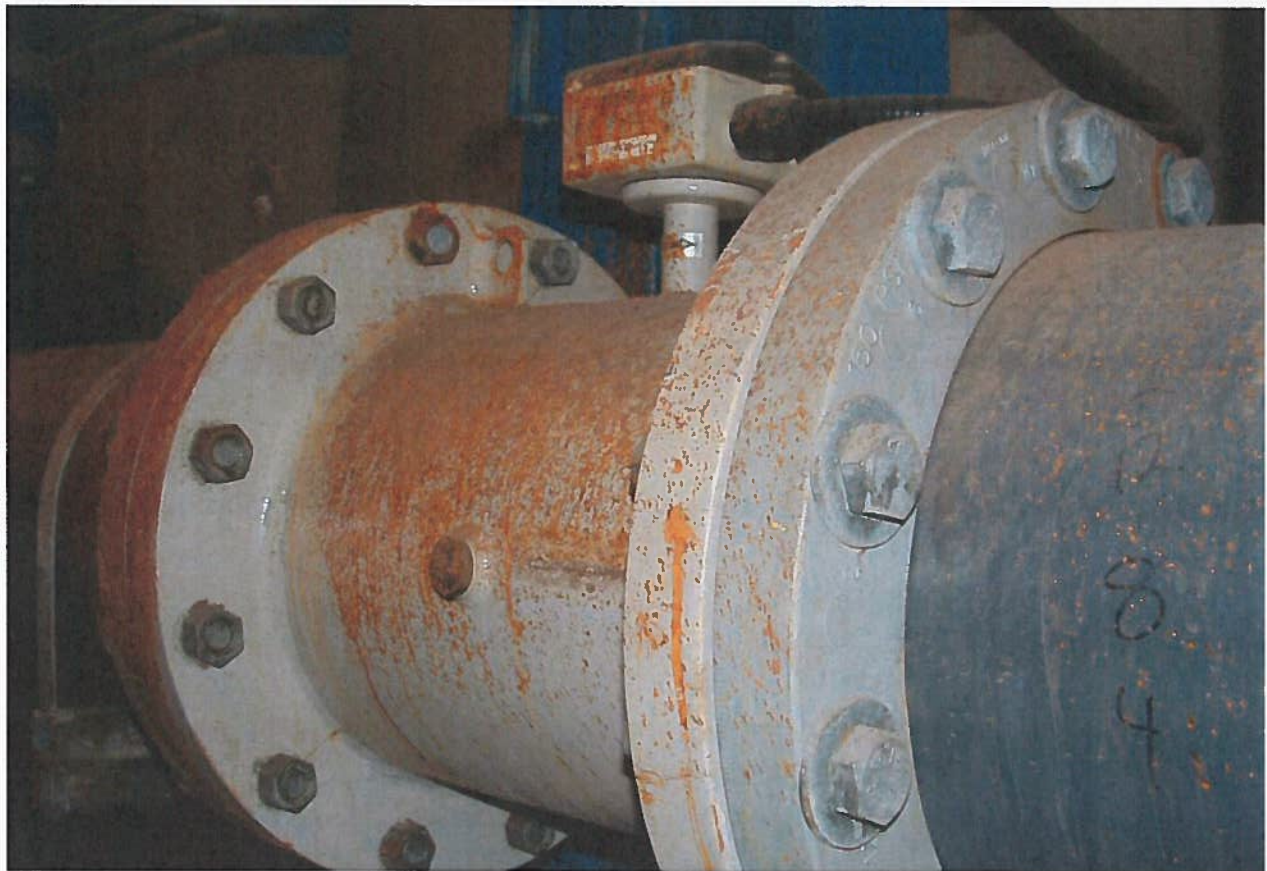
Wastewater treatment plant – 12-inch effluent flow meter for monitoring discharge to Purdam Drain
