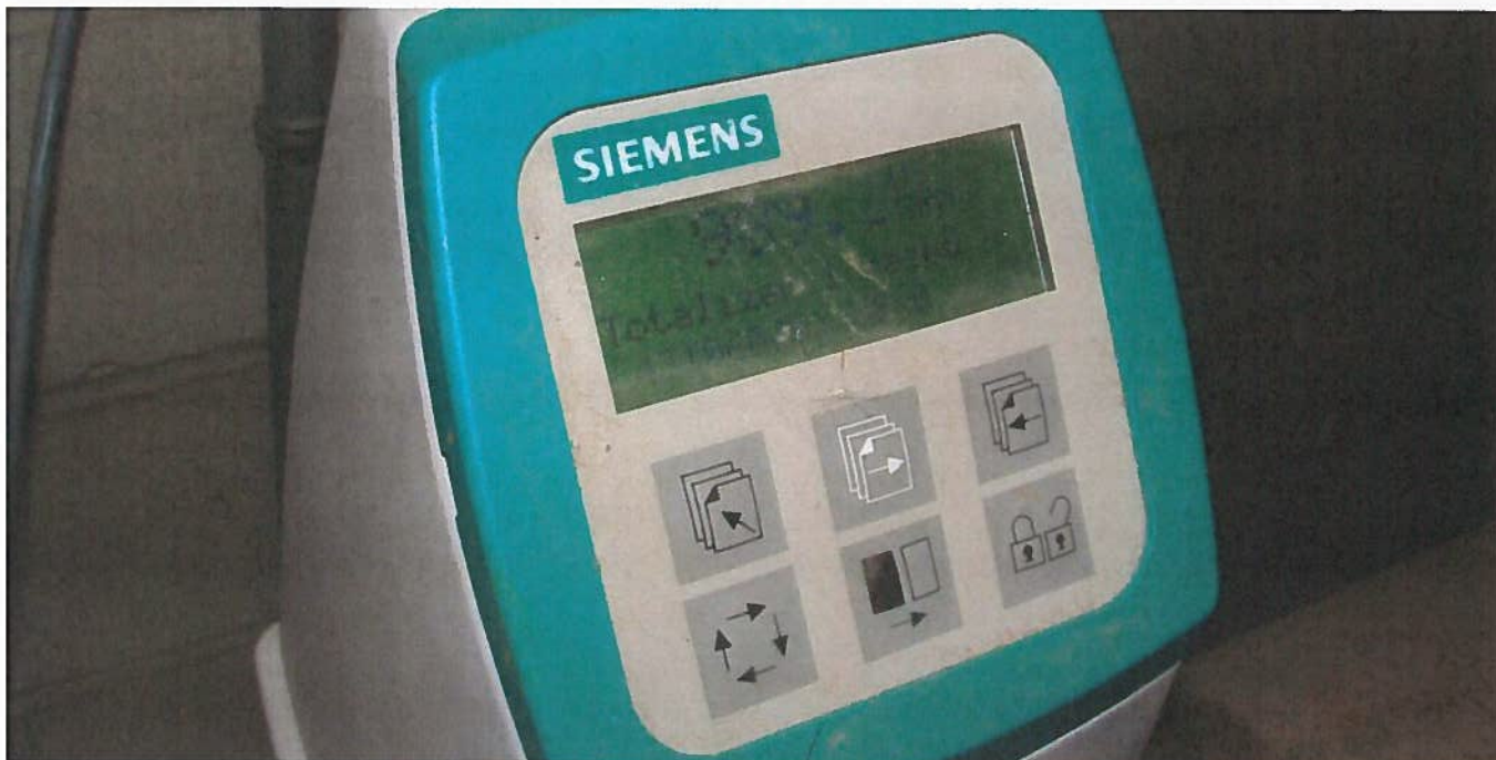
Well No. 2 flow meter display – 989 gpm
