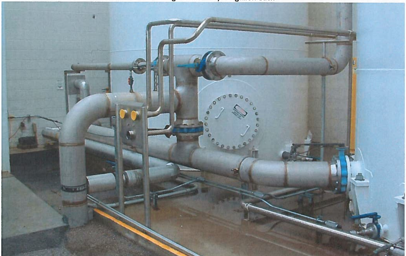
Inlet piping to water storage tanks and booster pumps
