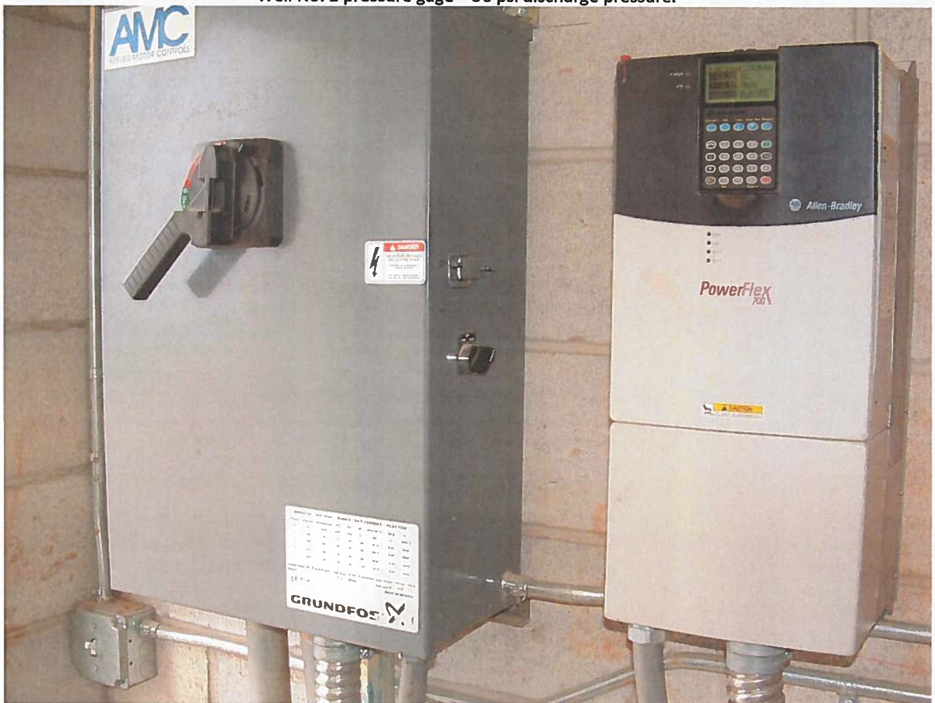
Well No. 2 motor controls. VFD operating at 60 hz.
