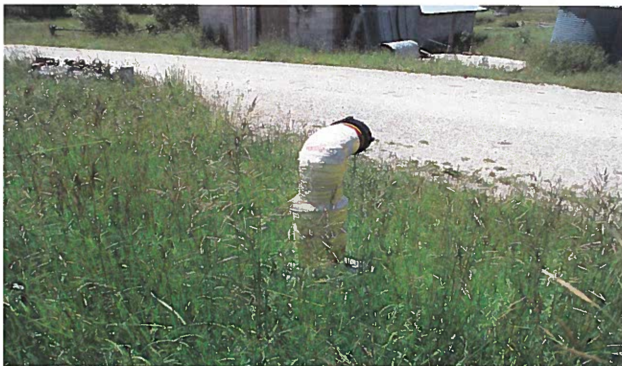
Dry Fire Hydrant just west of pond
