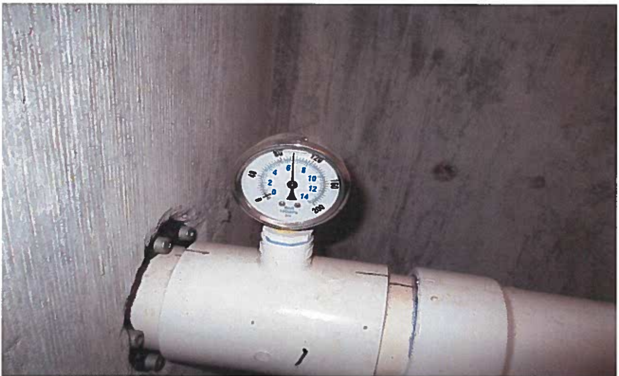
Pipe inflow to powerhouse
