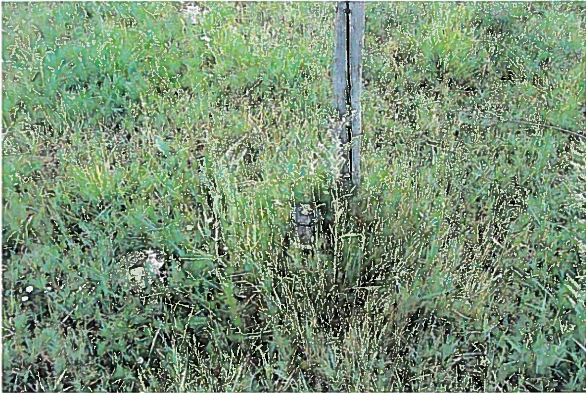
Riser by wooden post - water spraying near ground (system pressurized)
