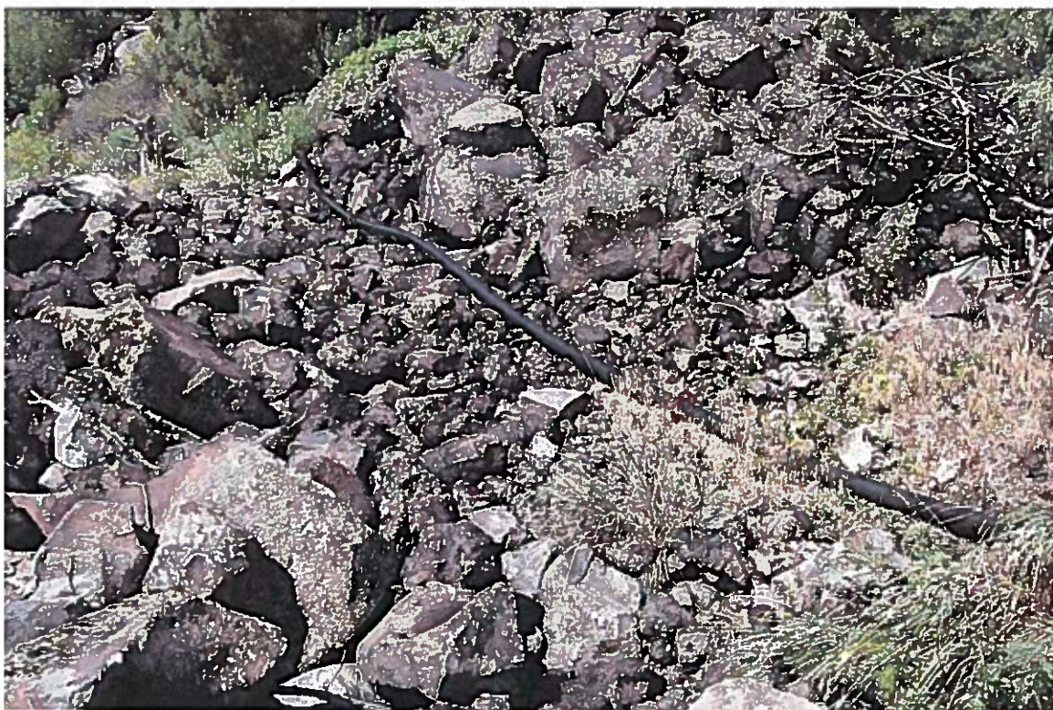
4-inch pipeline from spring to pond.
