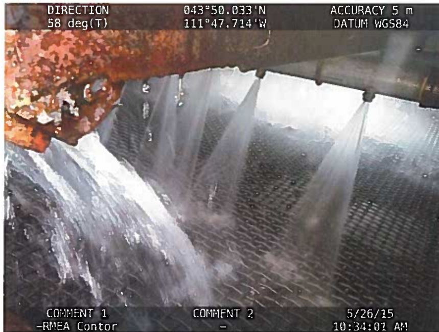
Photo IMG_0630.JPG. Spray jets below belting on upper screener.
