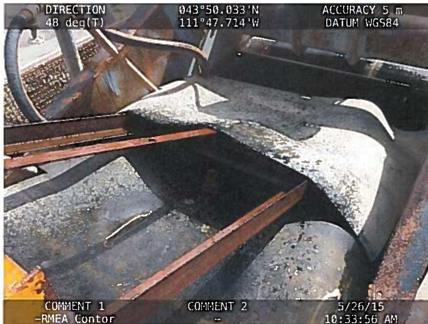
Photo IMG_0628.JPG. Looking down on belting shielding the spray on the upper screener. Spray was operational when photo was taken.
