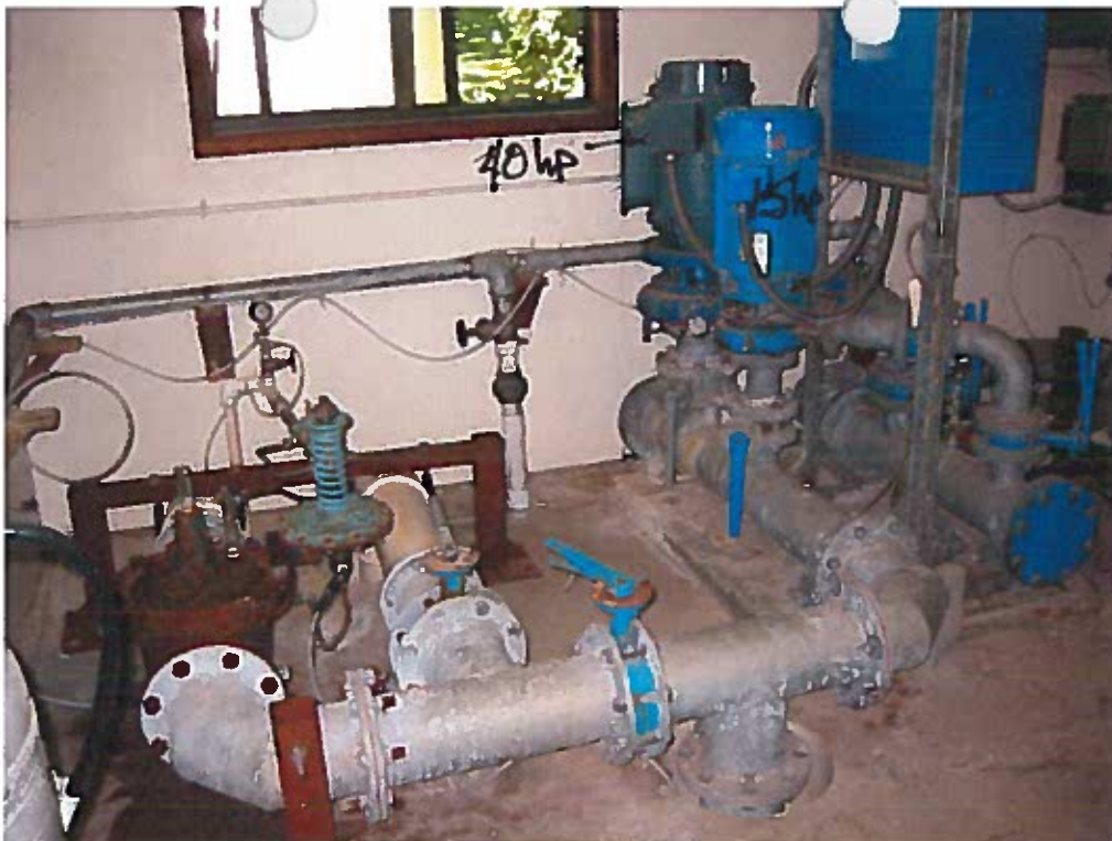
E, Plumbing Inside Pump House
