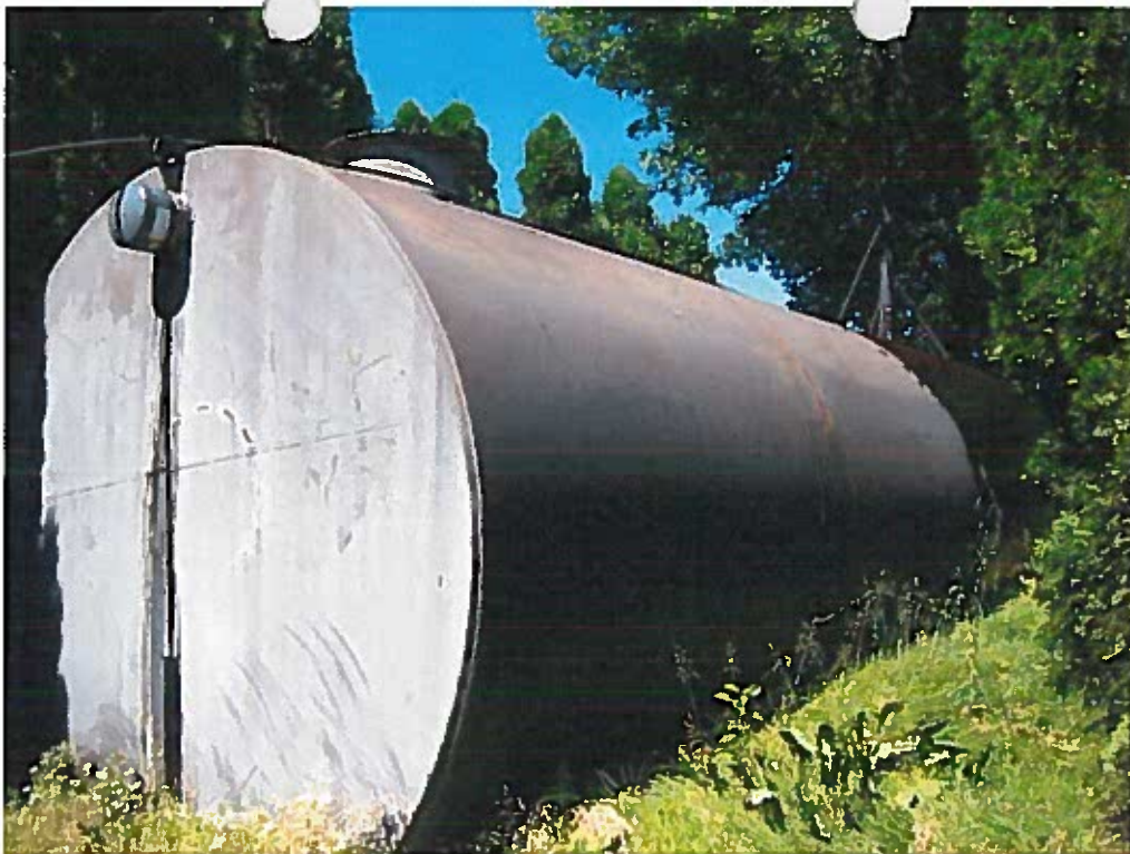
C. 15,000 Gallon Storage Tank Adjacent to Pump House
