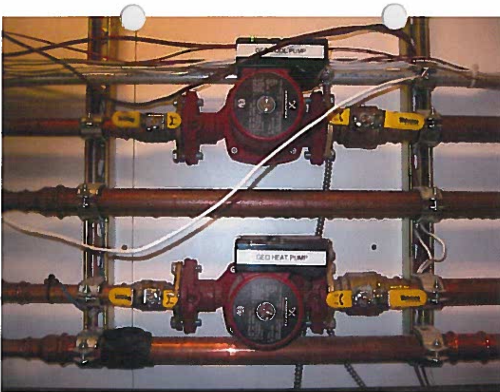
Heating and cooling plumbing inside utility room in home
