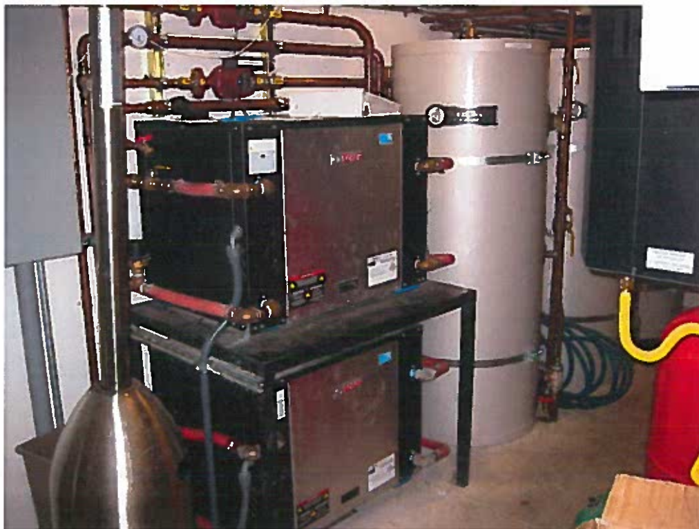
Heat pump units inside utility room in home
