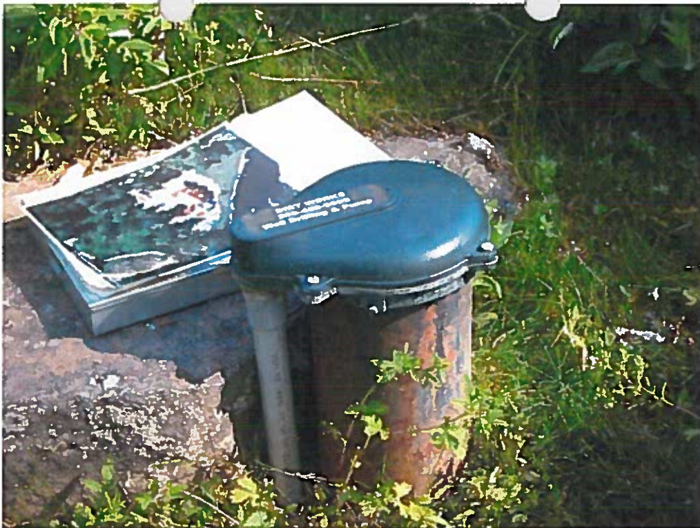
Heating and cooling extraction well – Point of Diversion
