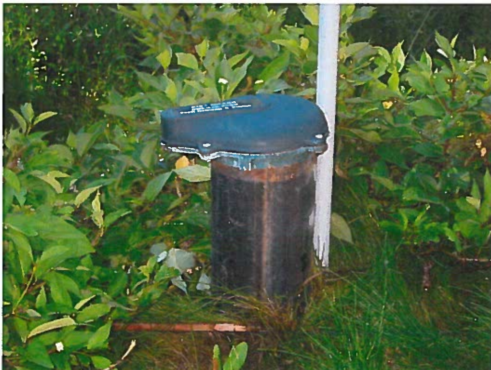
Heating and cooling injection well
