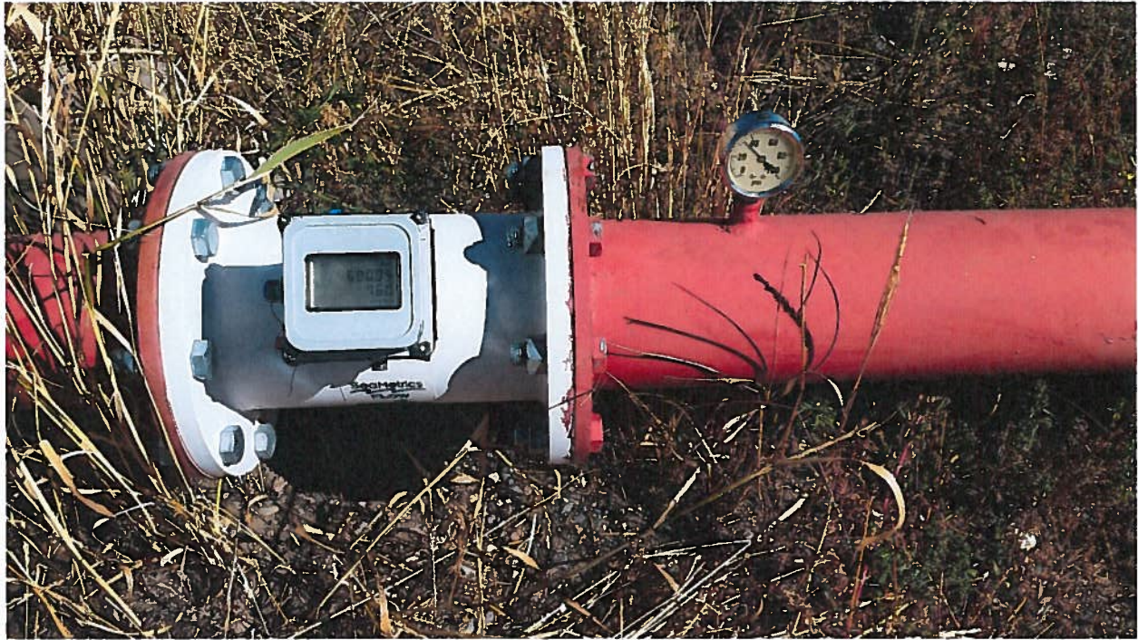
Response Photo 1: Flow Meter (680.05 acre-feet/760 gpm) and pressure gage (34 psi) during operation of 2 pivots with end guns and hand lines – prior to walking around site during operation
