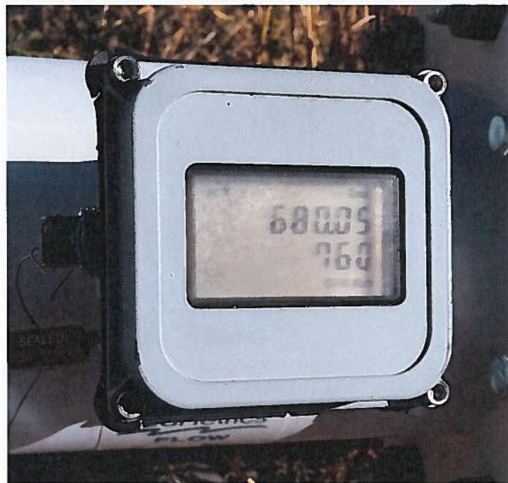
Response Photo 2: Close up of flow meter display
