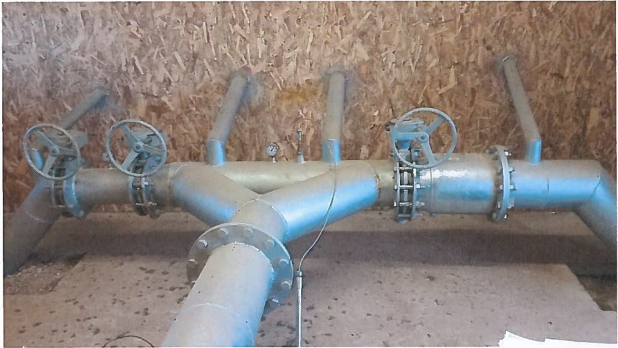
Photo 7: Photo of Pump Discharge Manifold. The south 10-inch branch (right) delivers water to the south pivot while the north 8-inch branch (left) delivers water for the industrial dust control and interconnects the well system.
