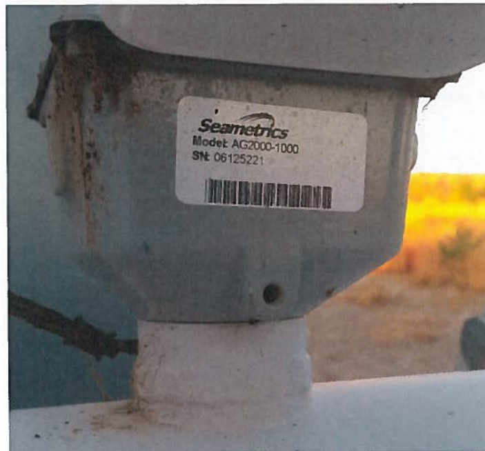
Photo 4: Photo of the installed Seametrics AG2000-1000 10-inch flow meter on the well discharge pipeline.
