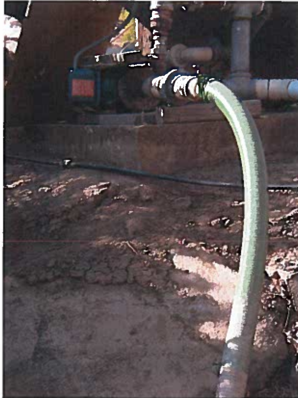
65-13739 Exam 9/14/2012: P/D motor and pump directly adjacent to check dam on Jackass Creek.
