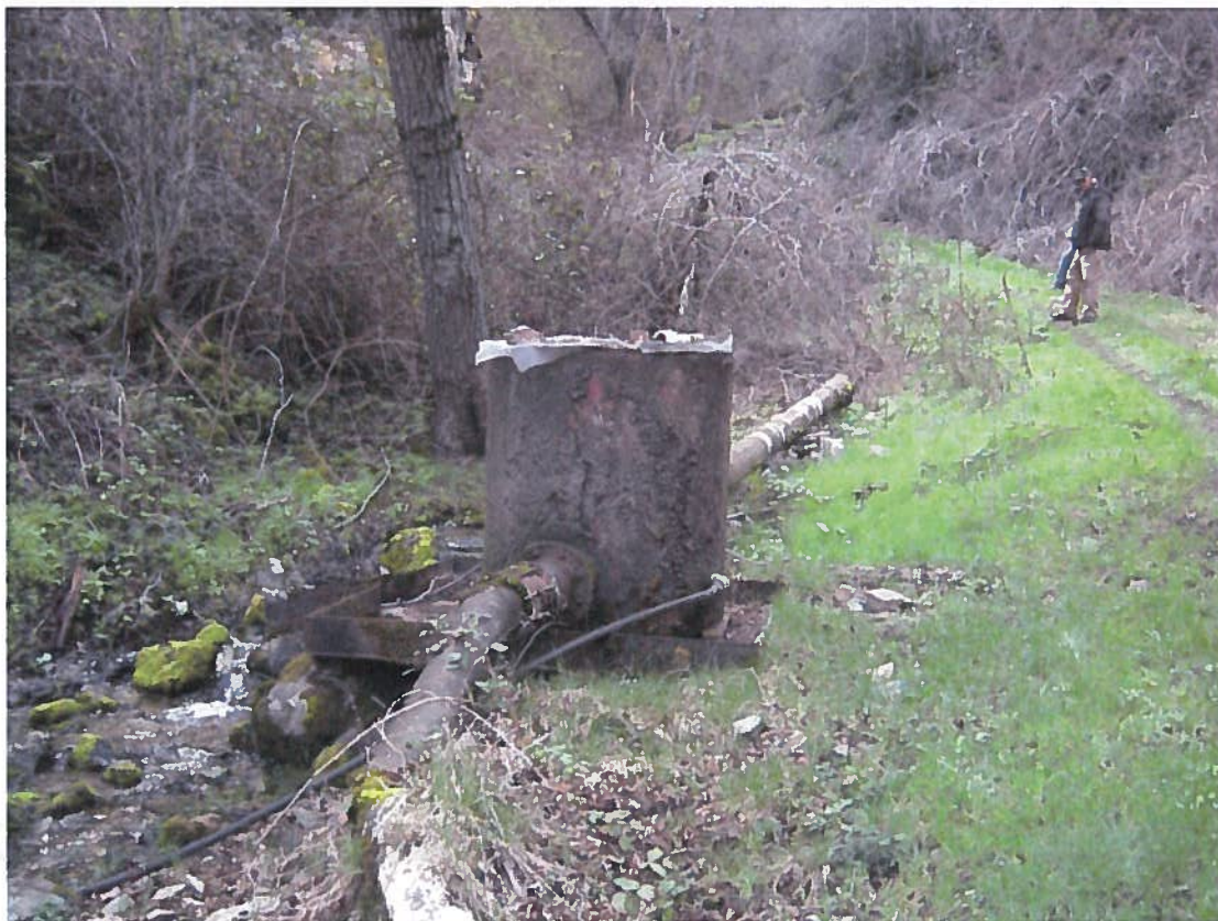
Figure 2 Pipeline from creek head gate to bubbler. Discharge pipe from bubbler in foreground.
