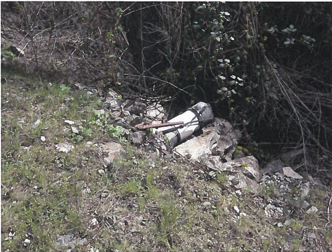
Figure 5 Pressure relieve discharge pipe and valve, discharges or spills water back to creek from mainline below bubbler.
