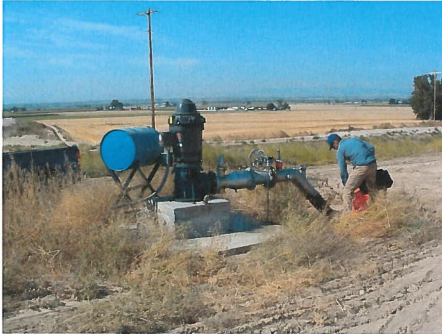
Figure 1: 16-inch Well and Vertical Turbine Pump
