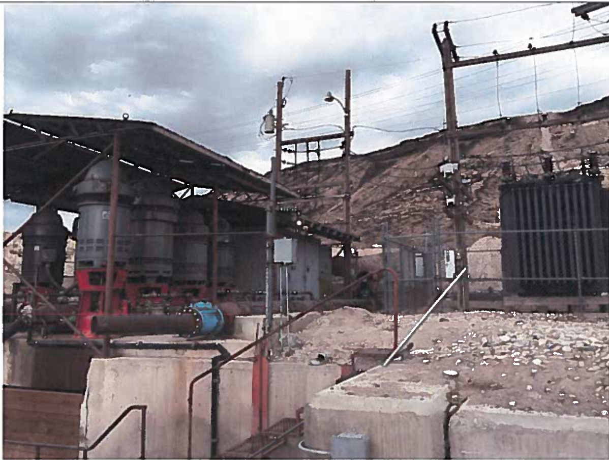
Pumping station. Pumps are lined in two rows of four. Water is delivered above ridge in photo.
