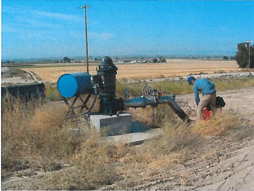
Figure 1: 16-inch Well and Vertical Turbine Pump
