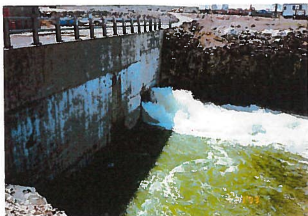
Discharge from powerhouse bypass, generators not on-line.
