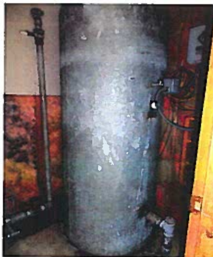
3. The only pressure tank for the system which can have air added manually.
