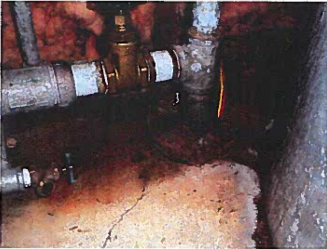
1. The wellhead located in the pump house and the height of it.
