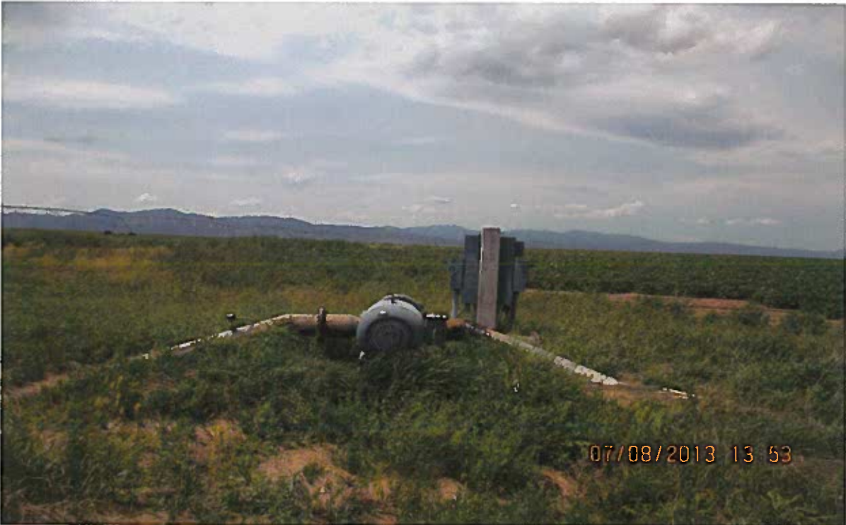
Booster Pump, looking West
