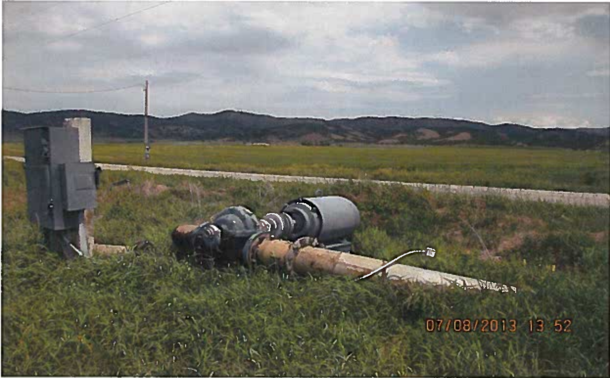
Booster Pump, looking Northeast
