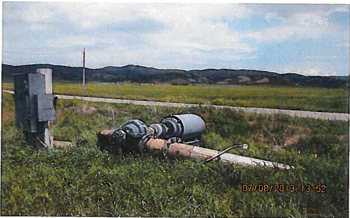
Booster Pump, looking Northeast
