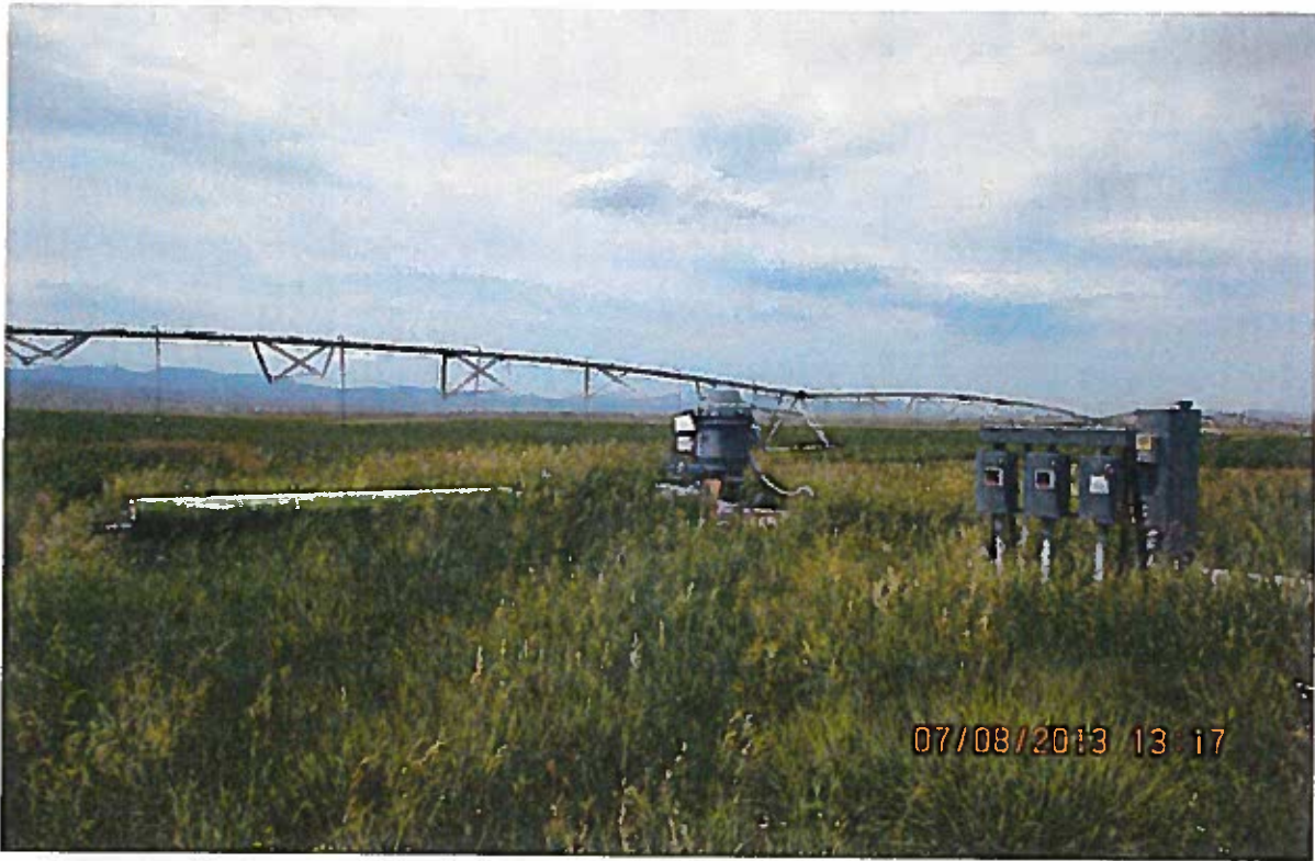
Well 3, looking Northwest
