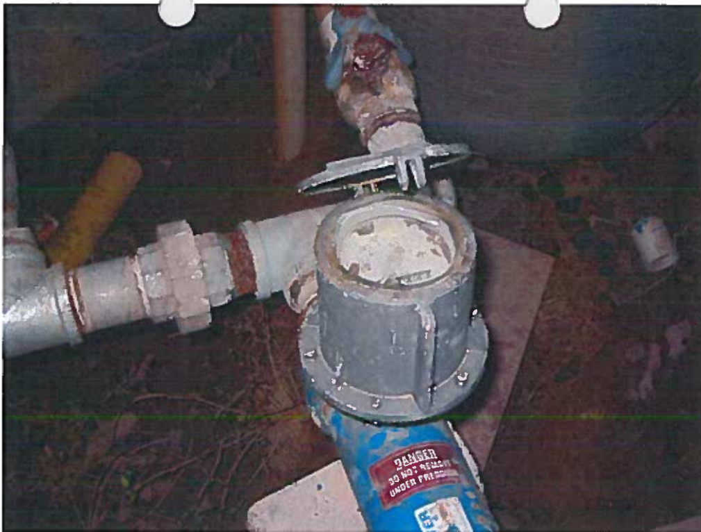
Flowmeter (not functioning at time of exam)
