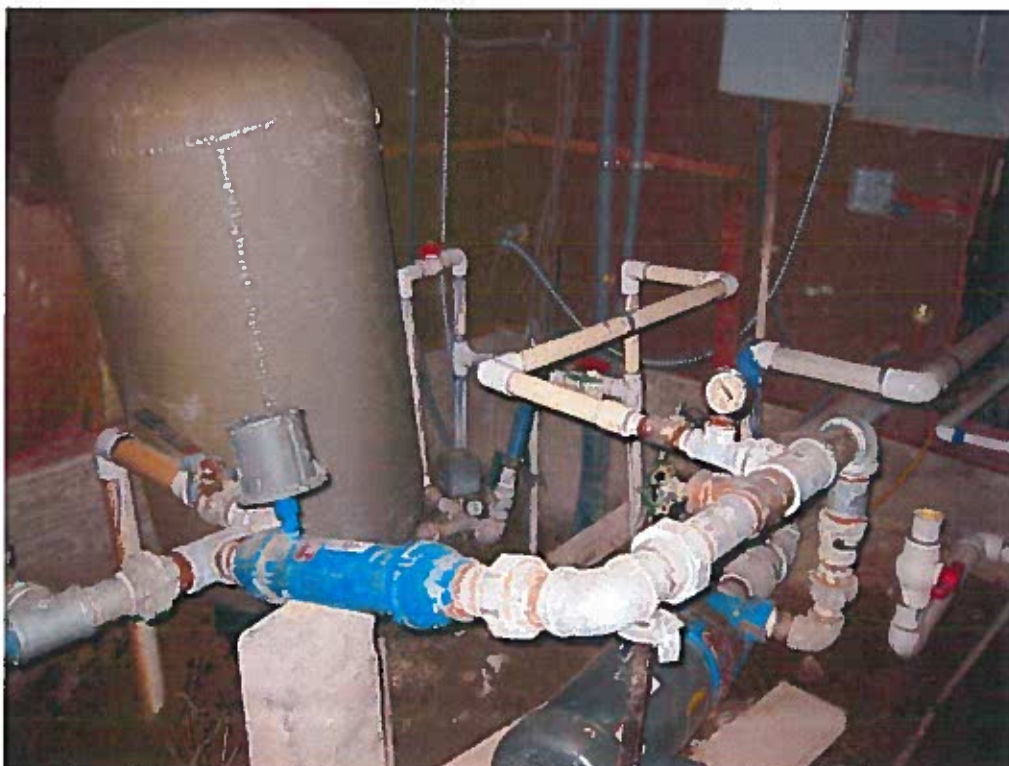
Plumbing Inside Pump House
