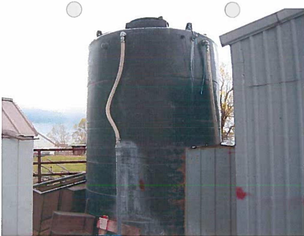
5000 Gallon Storage Tank
