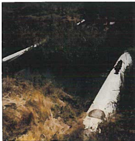
Mainline From Re-lift Pumps Across Feeder Ditch
