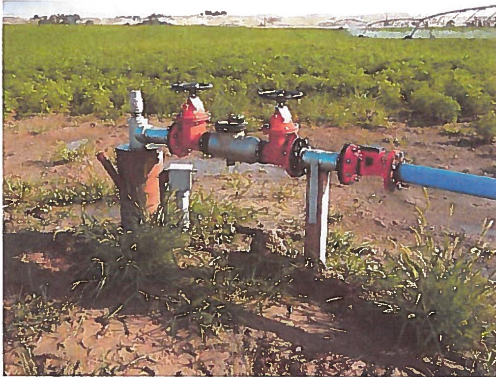
New well, valves and flow meter on the right
