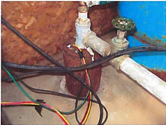
7. Well head for Well #2, shutoff and concern with the electrical wiring.
