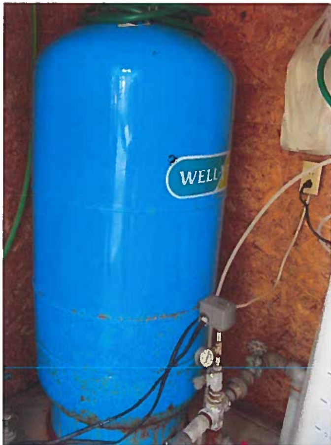
9. Pressure tank for Well #2.
