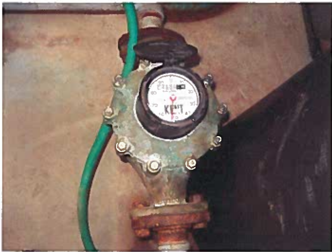
3. Flow meter in the pump house.
