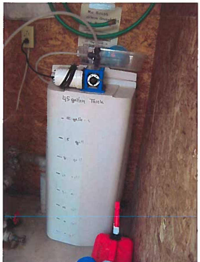
10. Chlorination system for the Back-up well.
