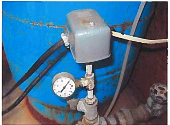
8. Pressure switch and broken pressure gauge for Well #2.
