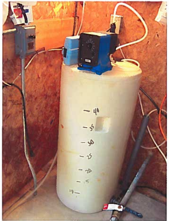
4. Chlorination system to the Main Well.
