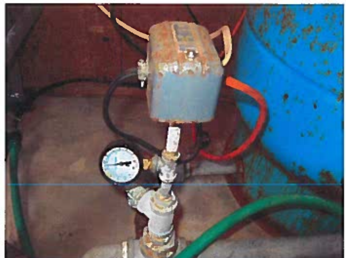
2. Pressure switch and gauge reading about 45 psi.
