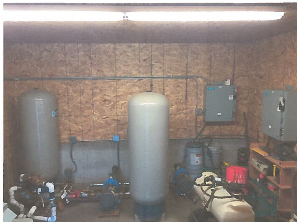
WELL ELECTRICAL, CONTROLS, BOOSTER SYSTEM AND PRESSURE TANKS
