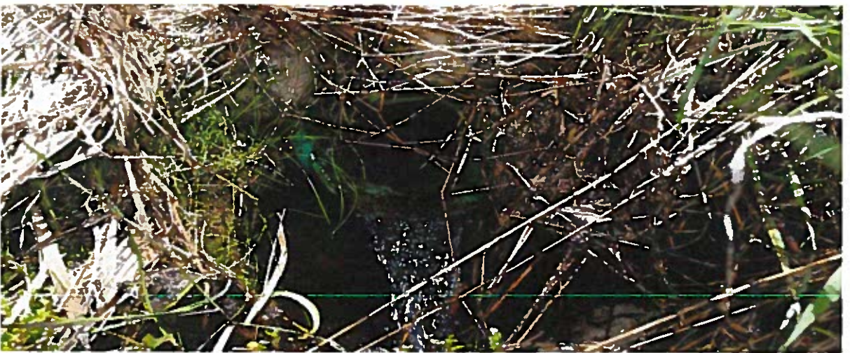
Pipe from spring
