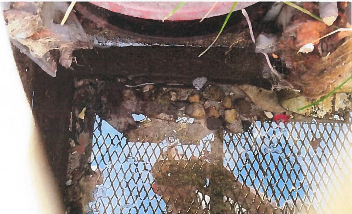
Photo 6: Looking into the NMID delivery box. Notice the NMID supply pipe entering the delivery box on the right and no NMID surface water entering the booster vault delivery pipe on the left.
