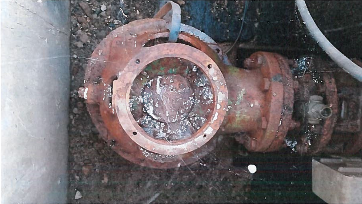
Photo 1: SWSW well located in a vault in East 2 nd Street. The well discharges groundwater into a 6-inch pipe to deliver water to a vault at the booster station in Storey Park.
