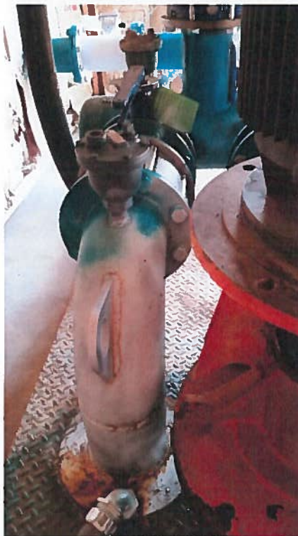
Photo 8: 25 hp submersible jockey pump inside booster station.
