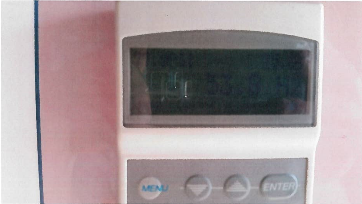
Photo 13: 53.8 Hz at 659 gpm and 77 psi discharge pressure. Set point for this system is 75 psi.
