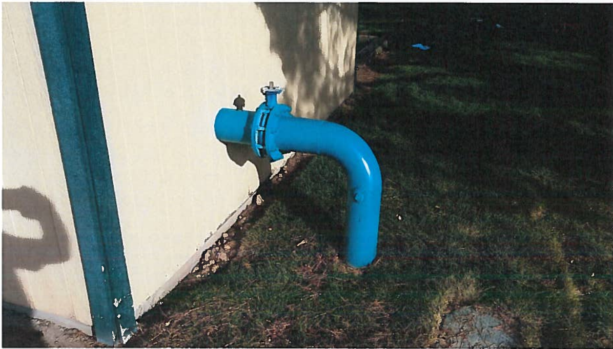
Photo 9: 6-inch steel discharge pipe exiting booster station and running underground to pressure sprinkler system.
