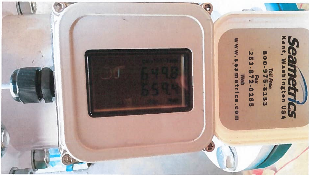
Photo 11: 6-inch Seametrics AG2000 flow meter showing instantaneous flow rate of 659.4 gpm.
