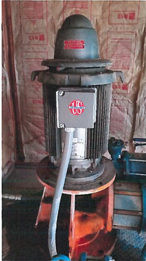
Photo 7: 25 hp VFD controlled vertical turbine pump inside booster station.
