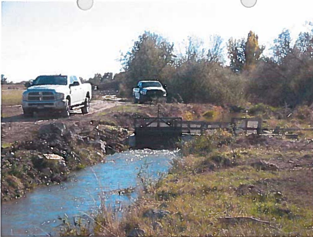
View looking upstream showing slide gate, fish screen, and POD
