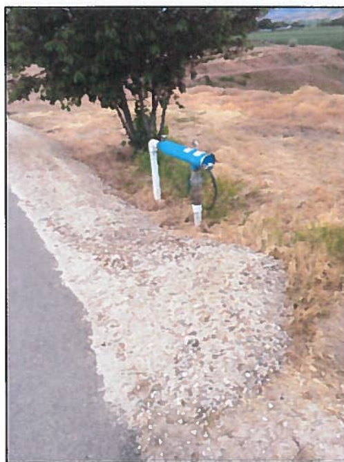
Filter for Pressurized Surface Water System T2N, R3W, S6, NWSE (Lot 11, Block 2)
