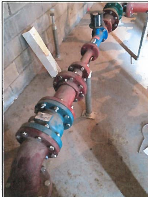
Piping from Well 2 & Flow Meter (inside pump house)
