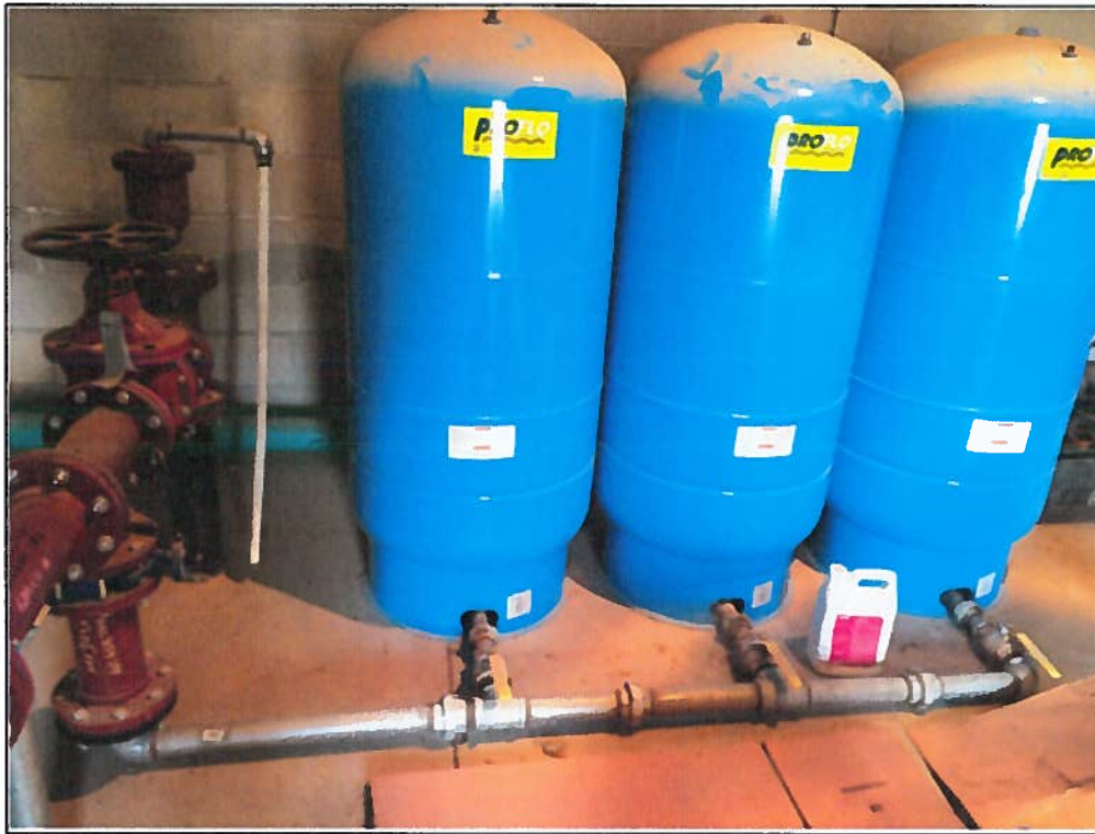
Pressure Tanks for Domestic Ground Water System (inside pump house)
