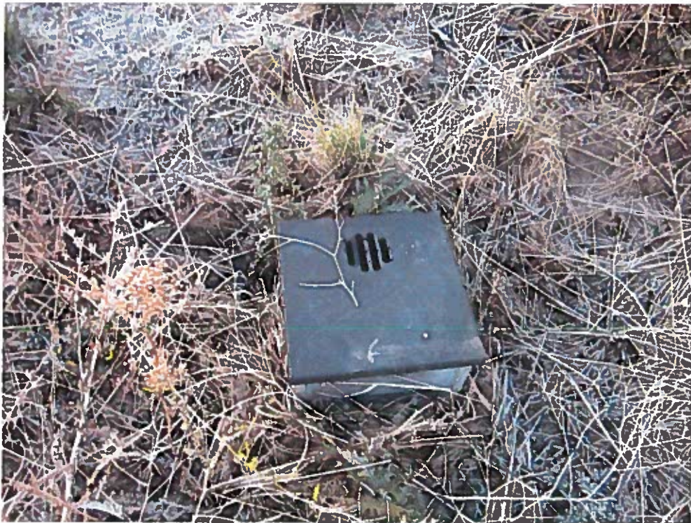
Figure 3: Water level control structure above outlet
