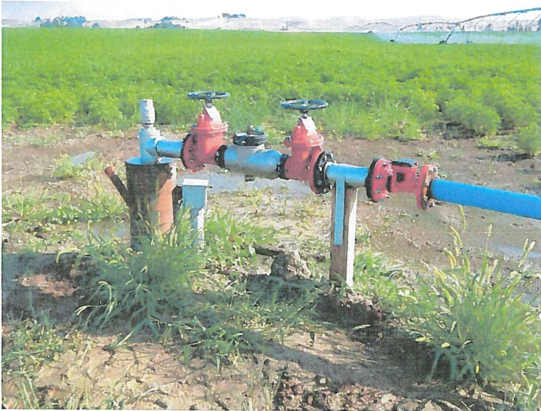
New well, valves and flow meter on the right
