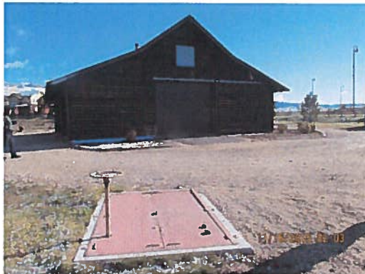
Secondary holding vault which gravity flows water into the pump house vault.
