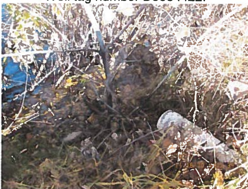
Plastic pipe which is used to discharge ground water from the well directly into the irrigation storage pond.
