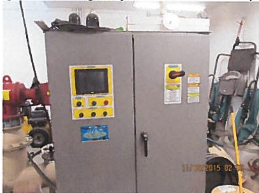
Pump room in the pump house.
