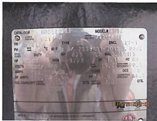
Pump label in the pump house.
