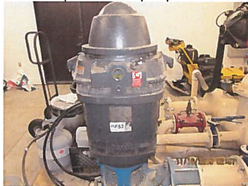
Pump in the pump house.
