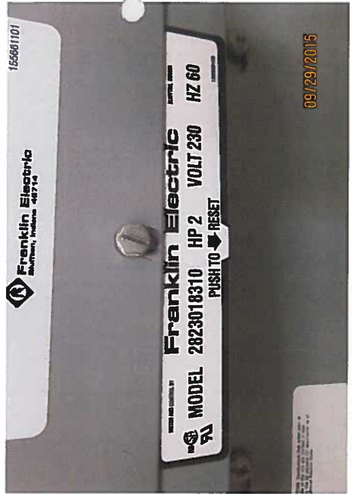
Pump in Well
