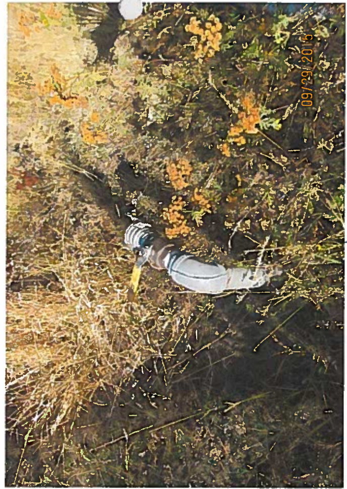
Fire Protection Line
