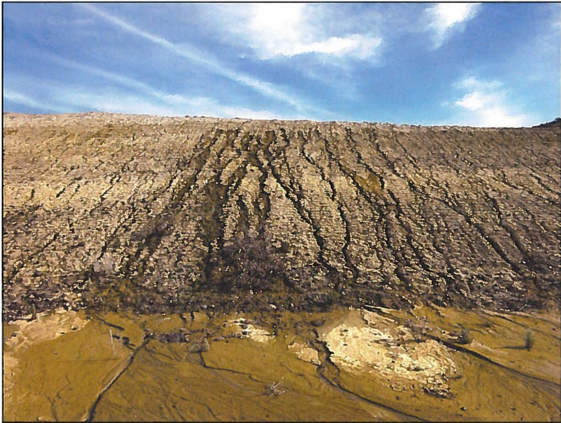
Photo 2 - Downstream, south-facing slope of the Diversion Dam located on Dry Creek. Flowing water was observed in some of the larger features; many of the smaller rills exhibited moisture.
