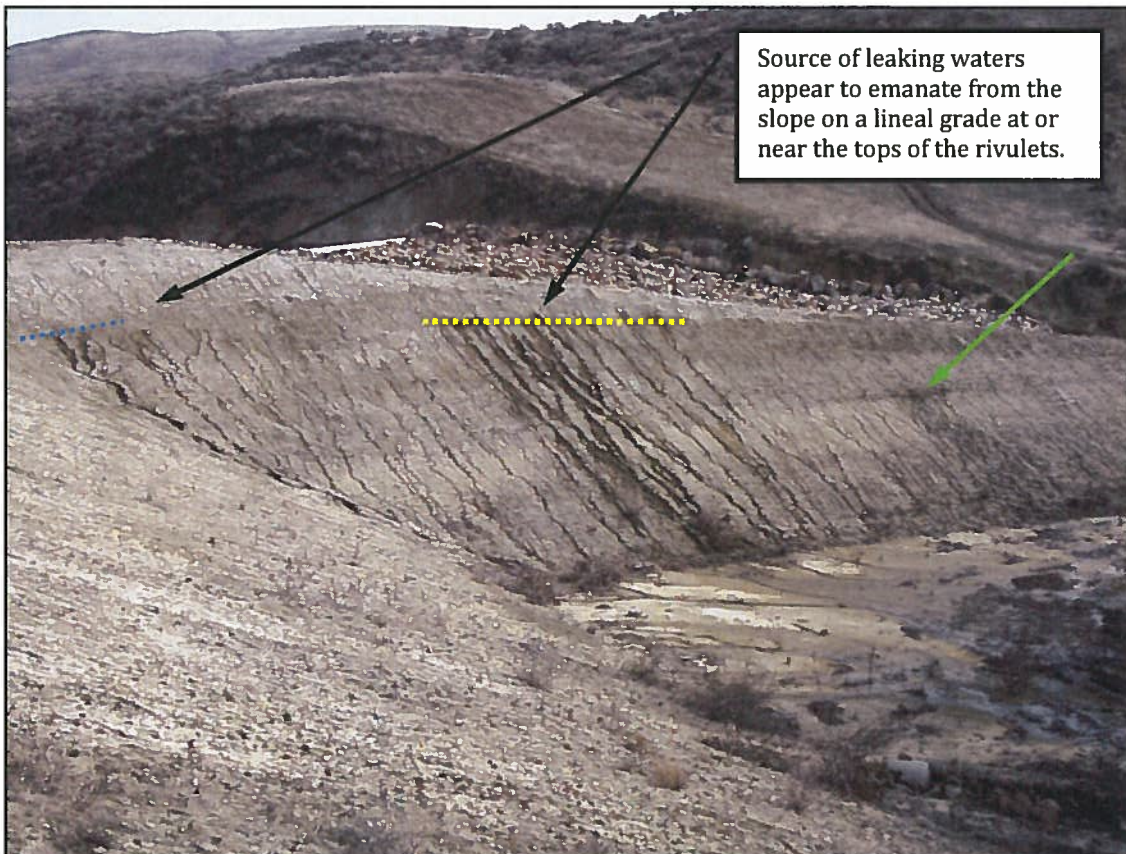
Photo 3 – Similar view illustrating the source of rivulets and deposited soil at the toe of the slope. Dry Creek Diversion Dam
