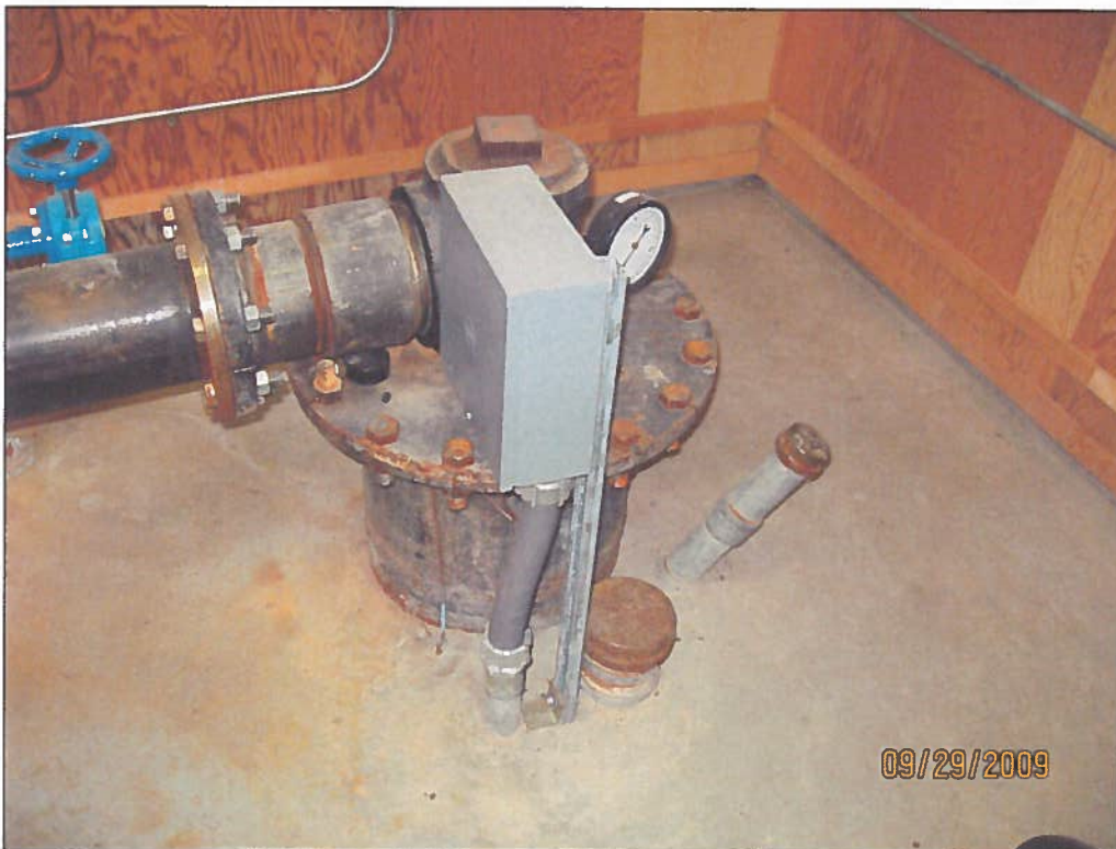
Figure 6: Well #2 well head and 6-inch discharge pipe to left.
