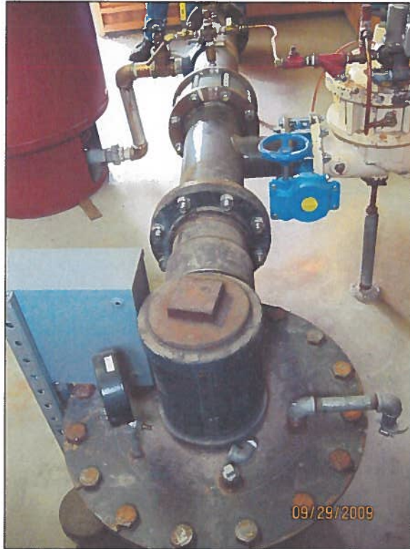
Figure 7: Well #2 discharge piping with flush control valve on right.
