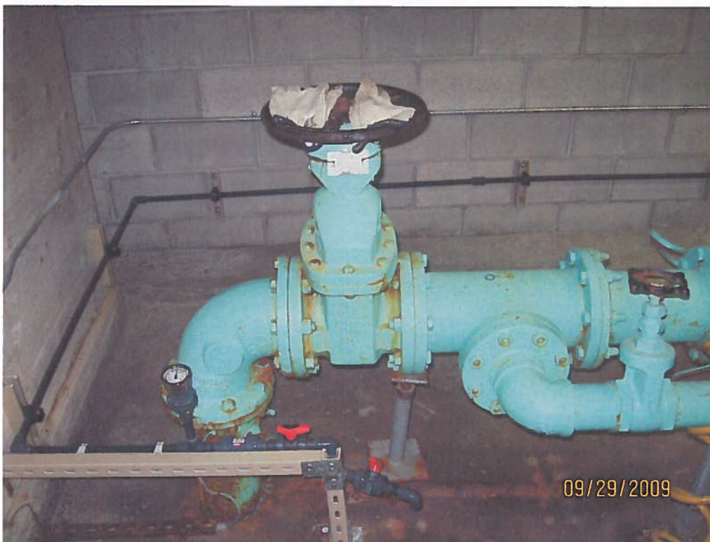
Figure 4: Well #1 discharges on left into municipal supply system.
