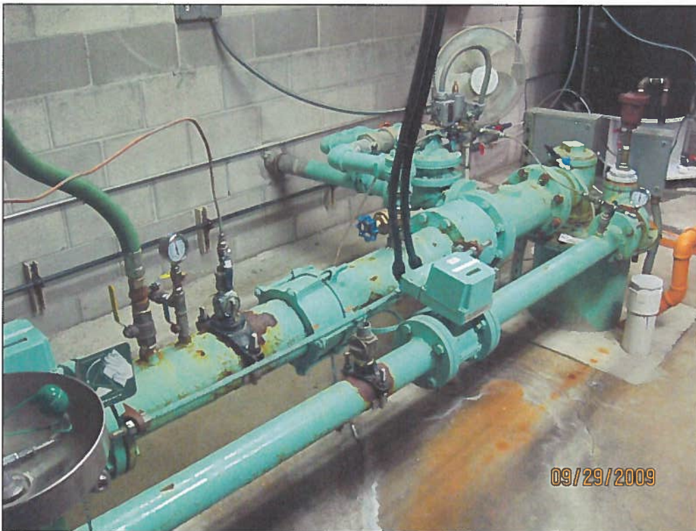
Figure 2: Well #1 with two discharge pipes with 6-inch mainline from 75-hp pump on left and 3-inch mainline from 25-hp pump on right.
