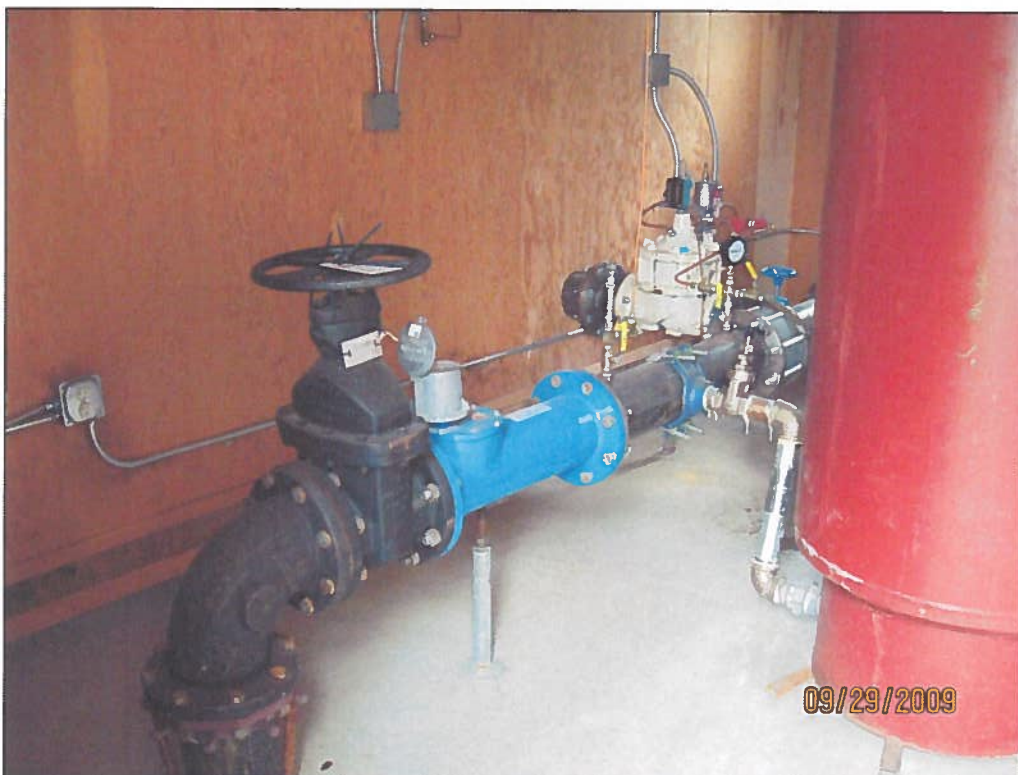
Figure 8: Well #2 discharge pipe with flowmeter (blue) and discharge to system on left side.
