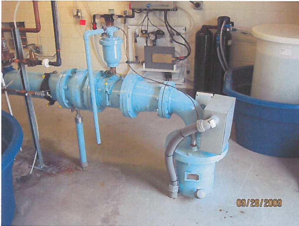
Figure 11: Well #3 and discharge piping.
