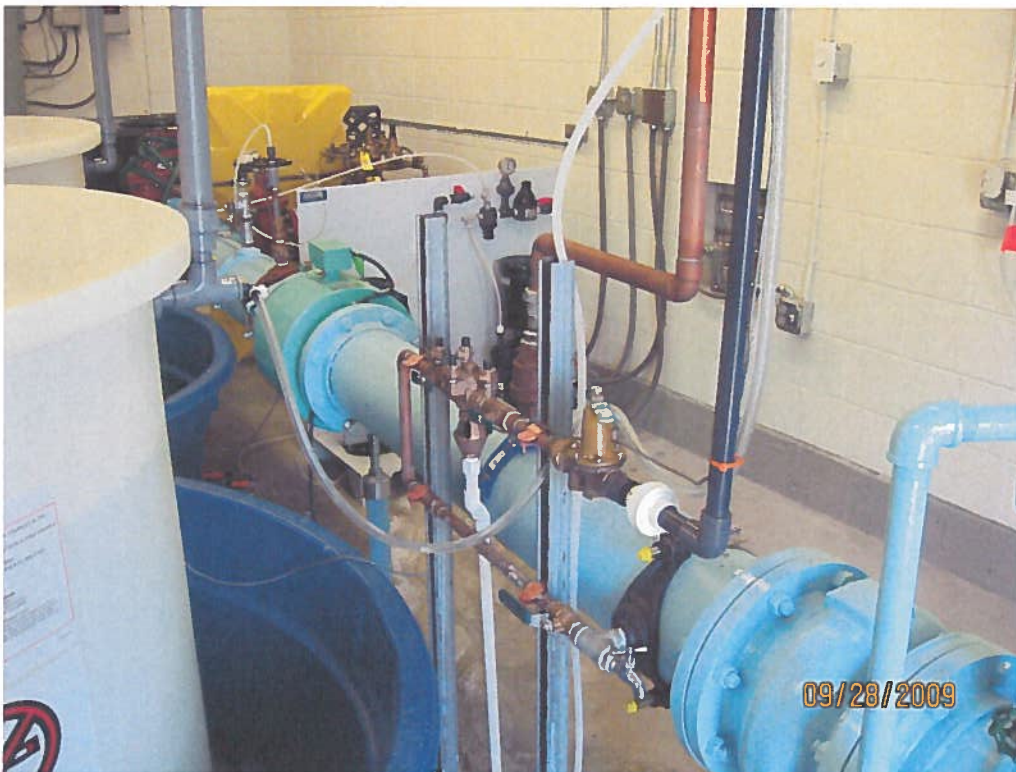
Figure 12: Well #3 discharge piping. Magnetic-type flowmeter is green and located left of photo center.
