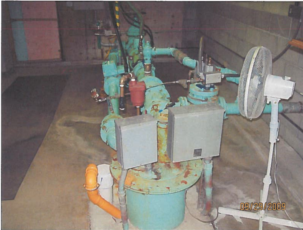
Figure 3: Well #1. Flush pipe discharges to outside of pump house on right.
