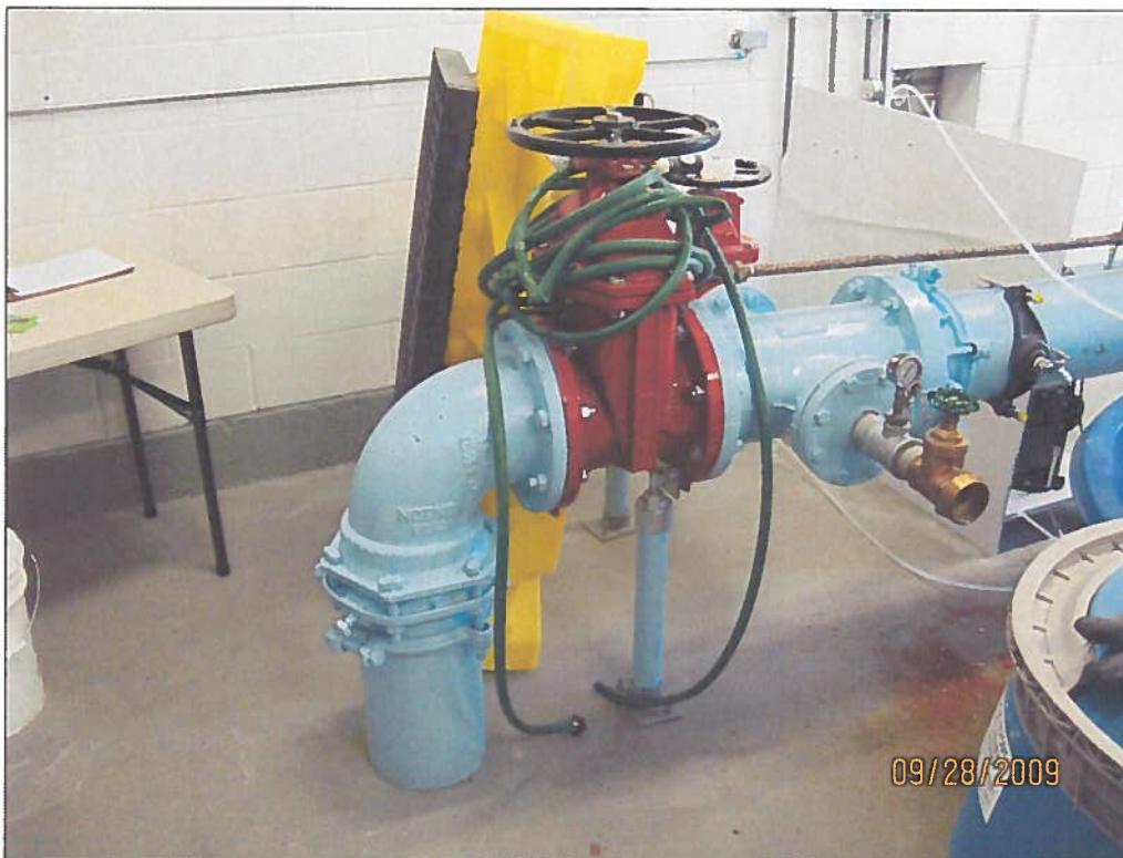
Figure 14: Well #3 discharge pipe into City's distribution system.
