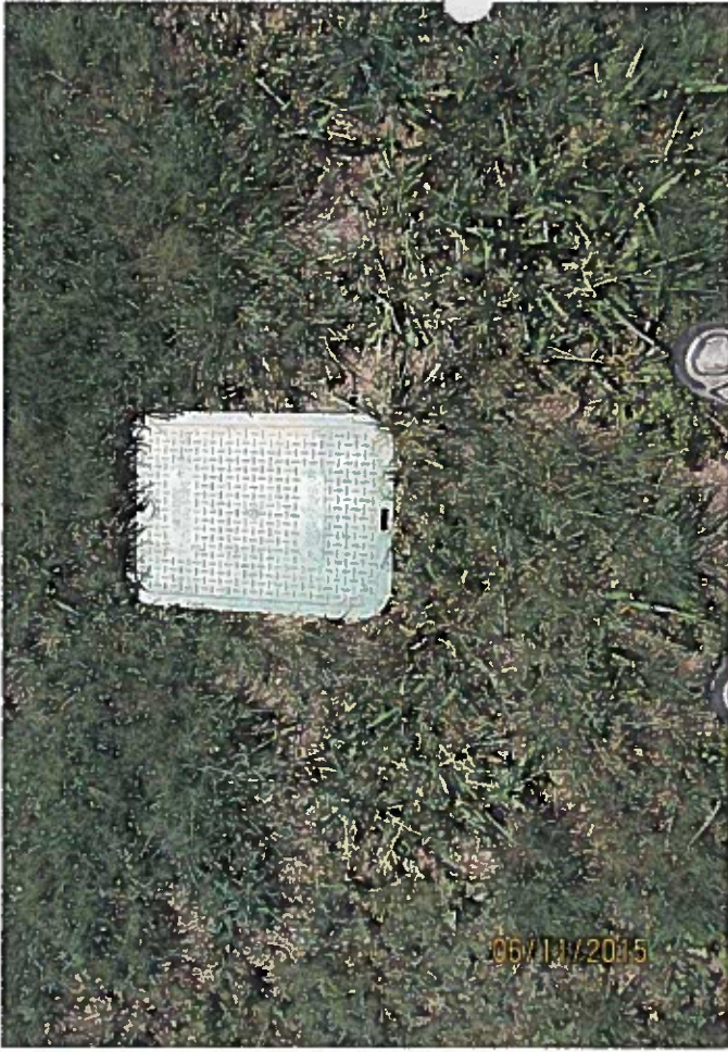
Control box Irrigation POU
