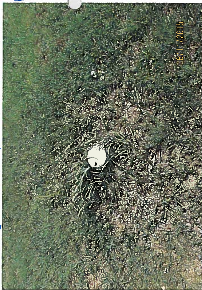
Pop up Sprinkler at POU
