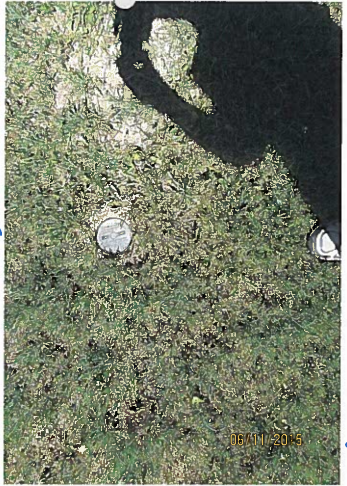
Pop Up Sprinkler Irrigation POU
