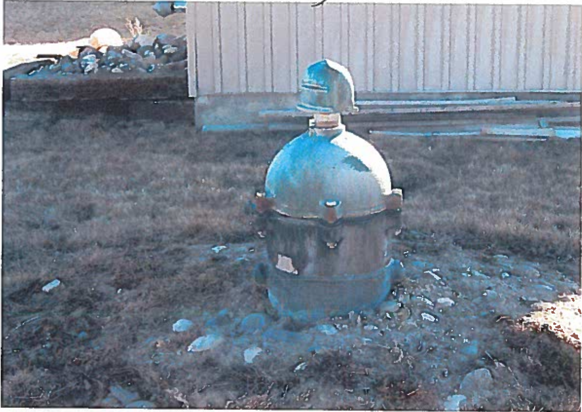
Well #3 (North well)
