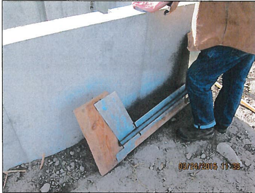
Figure 3: Two-foot Cipoletti weir before placing in concrete weir box. Locking headgate is installed upstream of this weir box.
