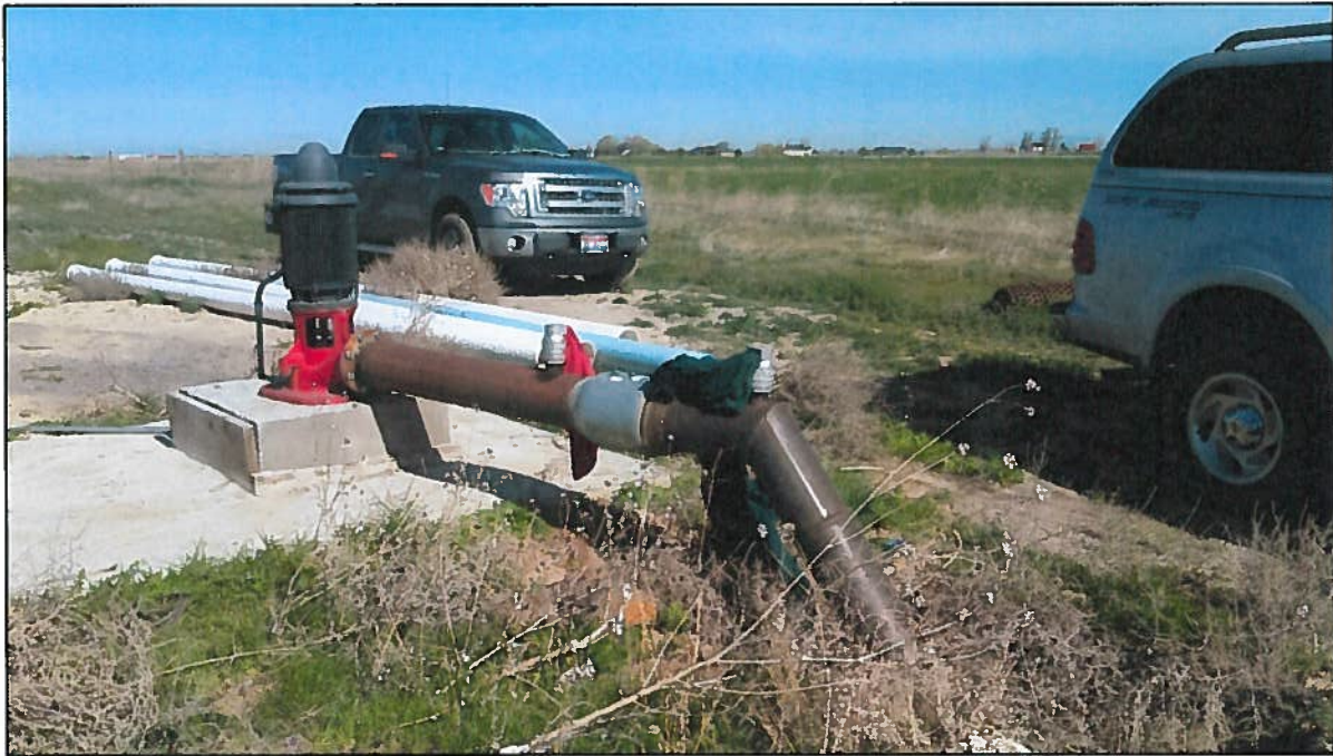
Figure 1: Well is equipped with 30-hp motor and vertical-turbine pump.
