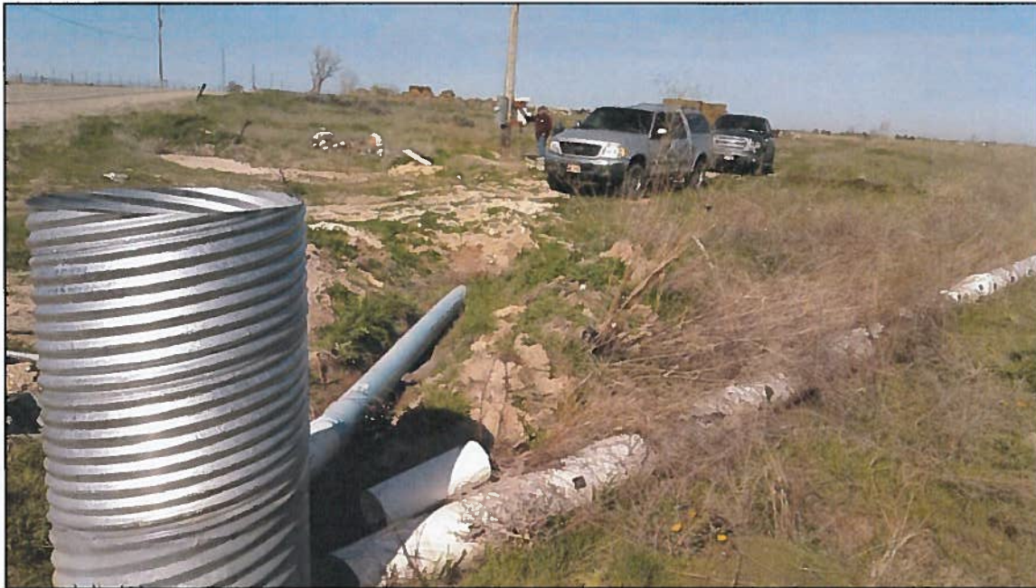
Figure 3: Flow enters CMP standpipe where it is directed to a gated pipeline (NW) or ditch (E).
