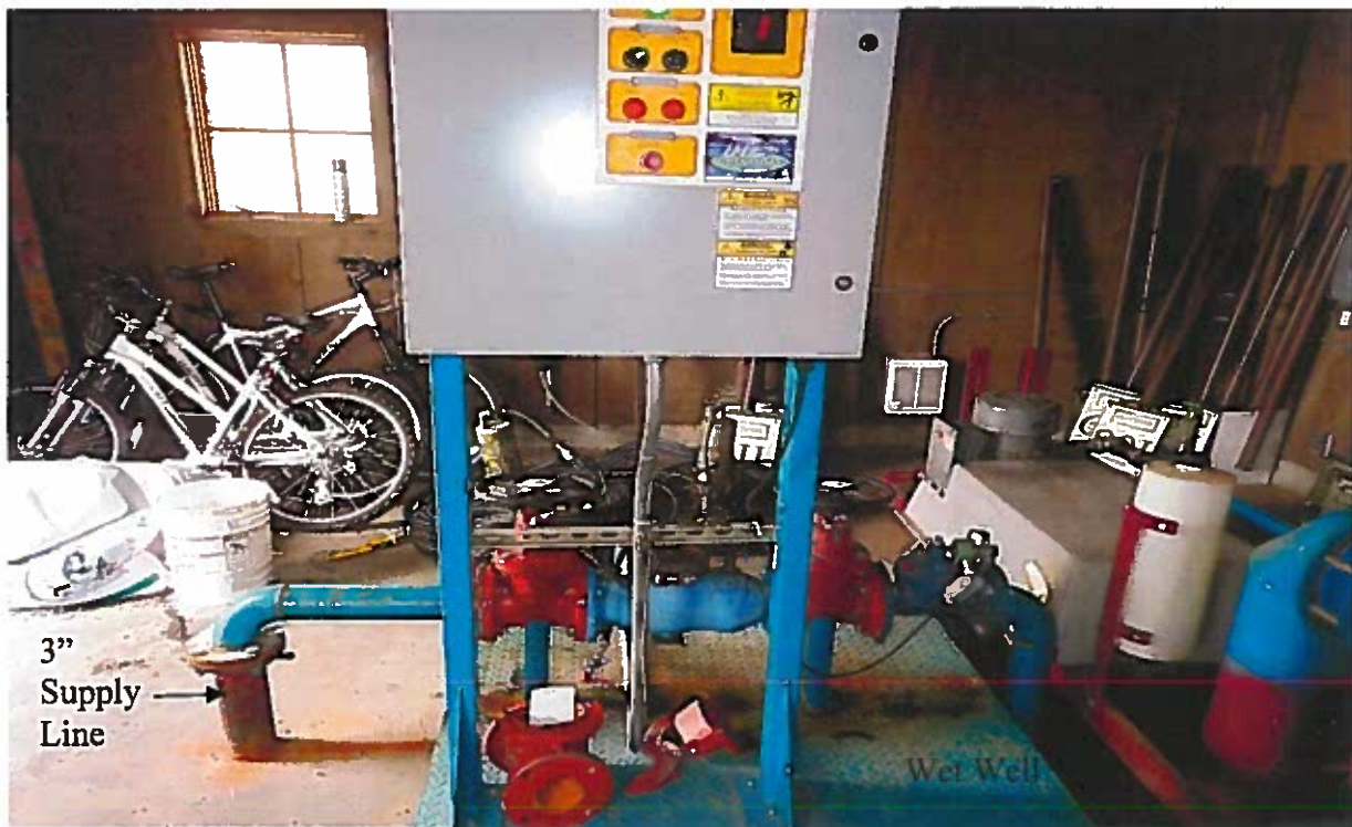
View of the control panel, 3" supply line from Well No.1, and the wet well located in the irrigation pump house.
