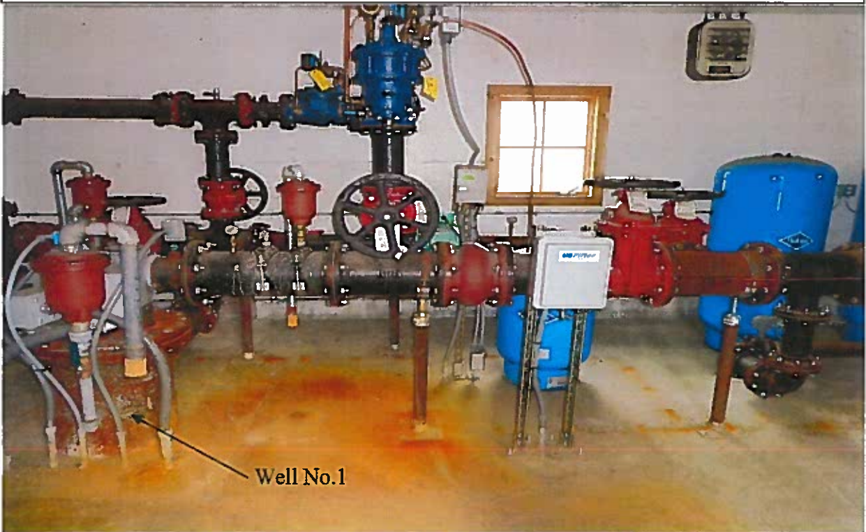
Point of Diversion: View of Well No.1 and the 20" well casing, piping, and appurtenances. The well/pump house for Well No.1 includes the main discharge and distribution main lines to the development and to the pump house adjacent to the storage ponds.
