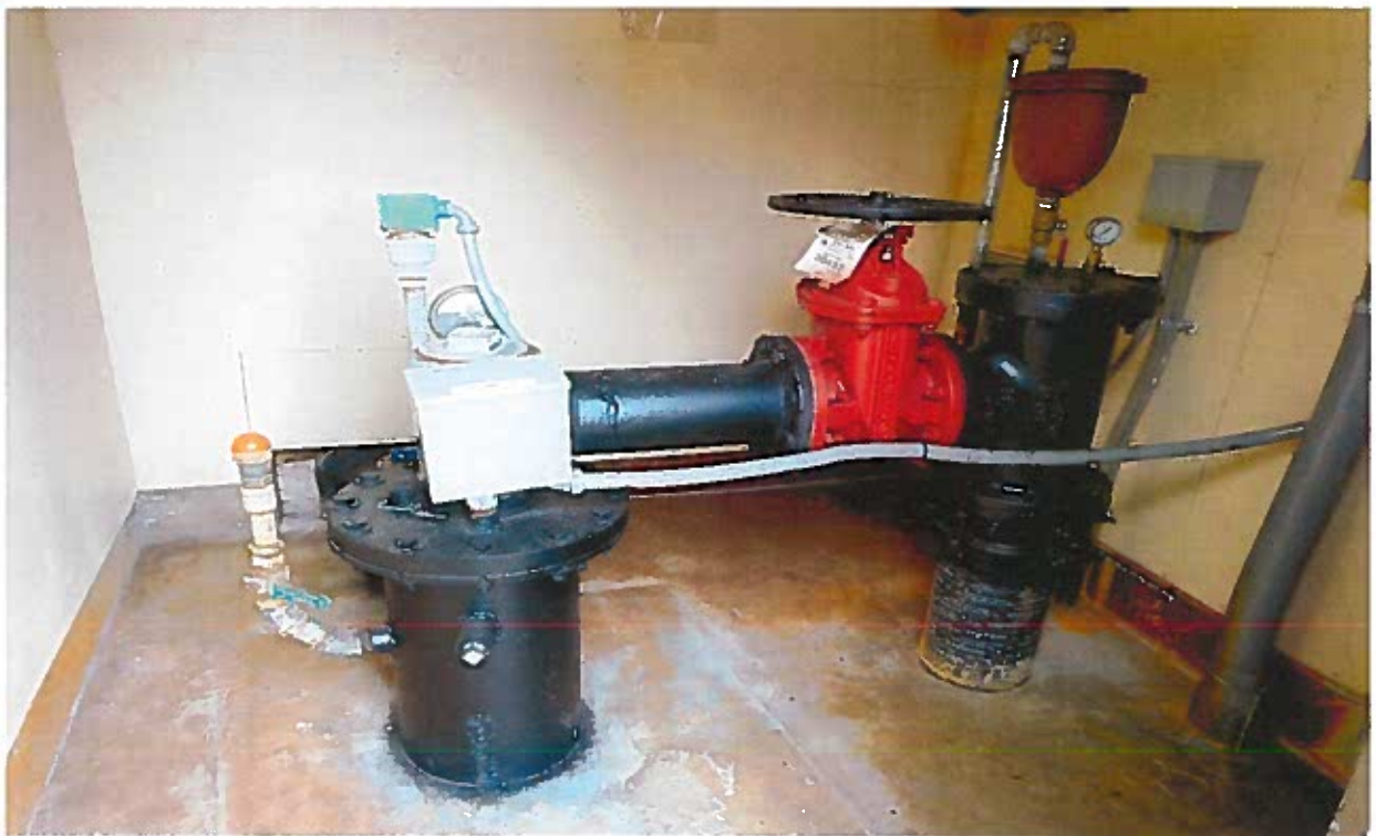
Point of Diversion: View of Well No.2 and the 12" steel casing in the small well/pump house west of the lodge building.
