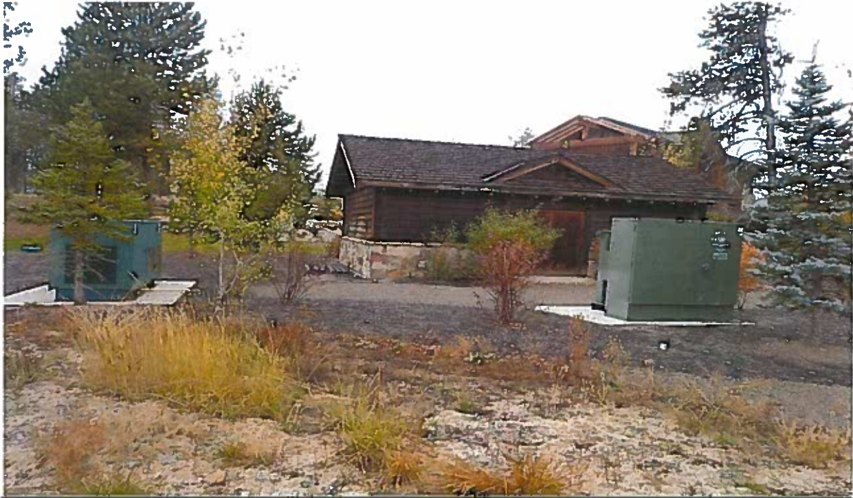
Point of Diversion: View westerly of the well/pump house for Well No.1. Well No.1 is the main well used to maintain the water surface elevations for the two storage ponds. A second well, Well No.2, is a backup groundwater source for the development.
