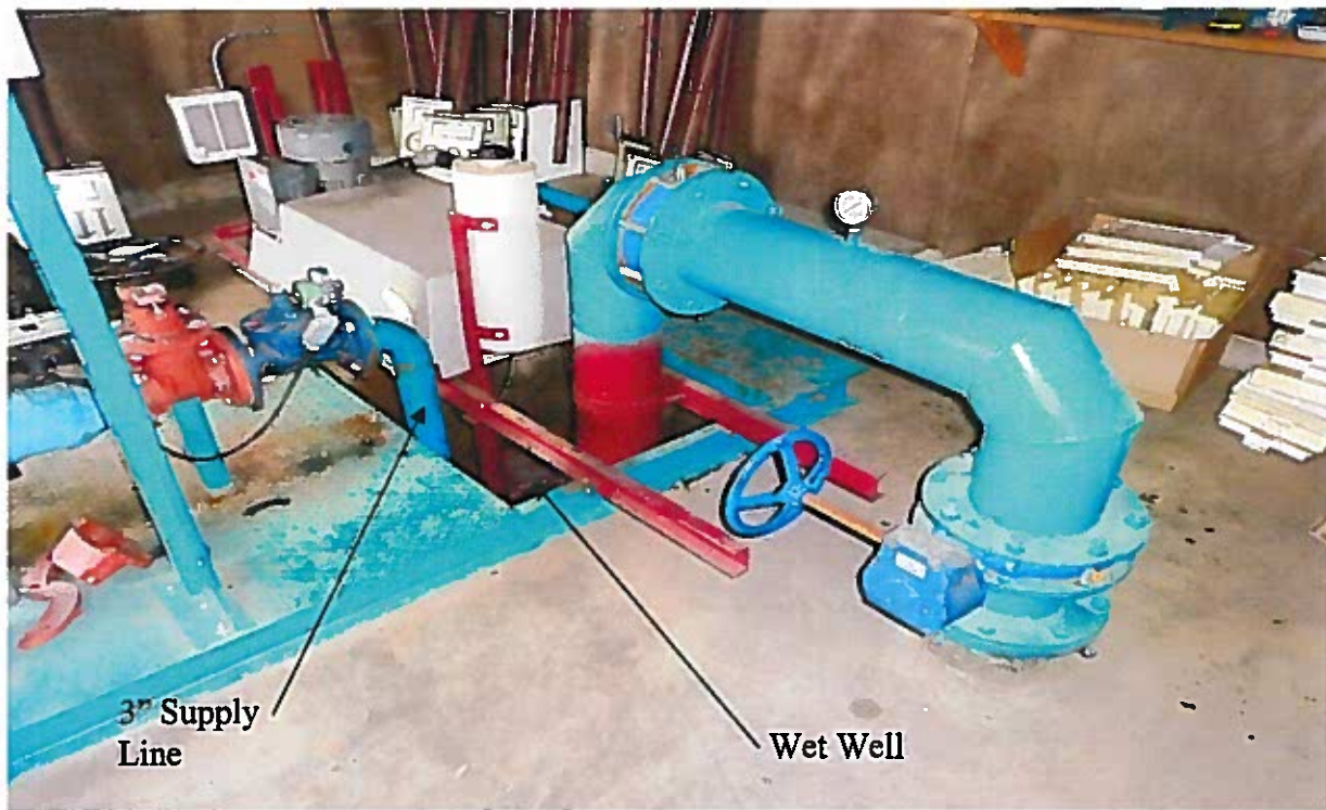
View inside of the irrigation pump house of the 3" supply line from Well No.1, the irrigation wet well, and the irrigation discharge main line. Water is pumped from the wet well to the storage ponds to replace the water losses due to evapotranspiration and leakage.
