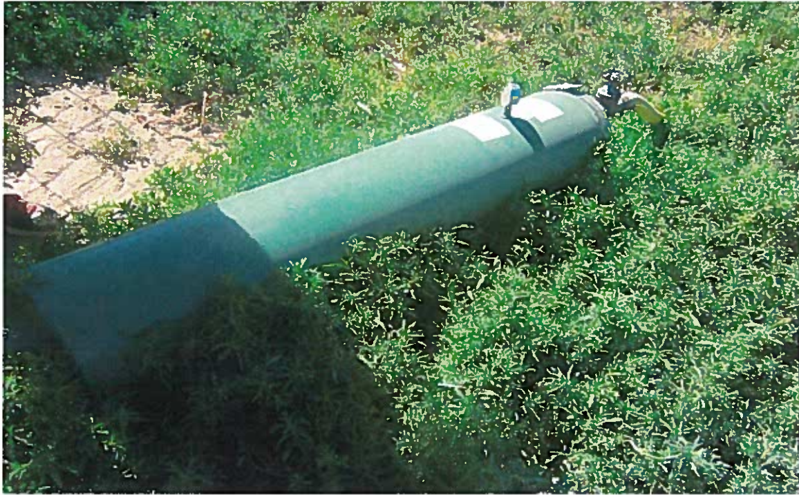
Past the filter, water is diverted through 4" buried pipe, seen here at the right end of the filter.
