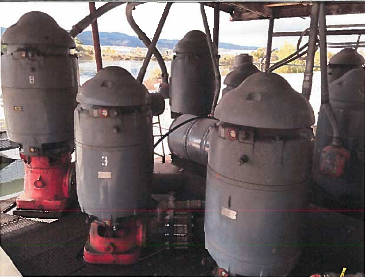
Pumps are lined in three rows of three, 9 pumps total, labeled as shown. (There is no No. 7)
