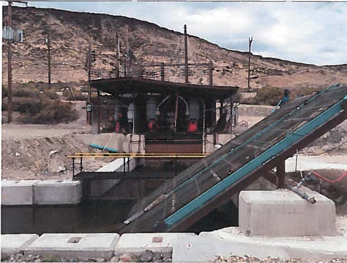
Pumping station looking north. Water is delivered above ridge in photo.
