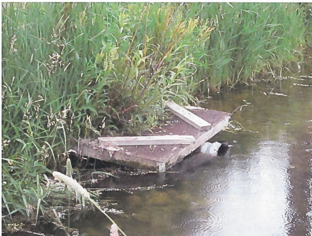
Diversion from large pond to the L7 Ditch
