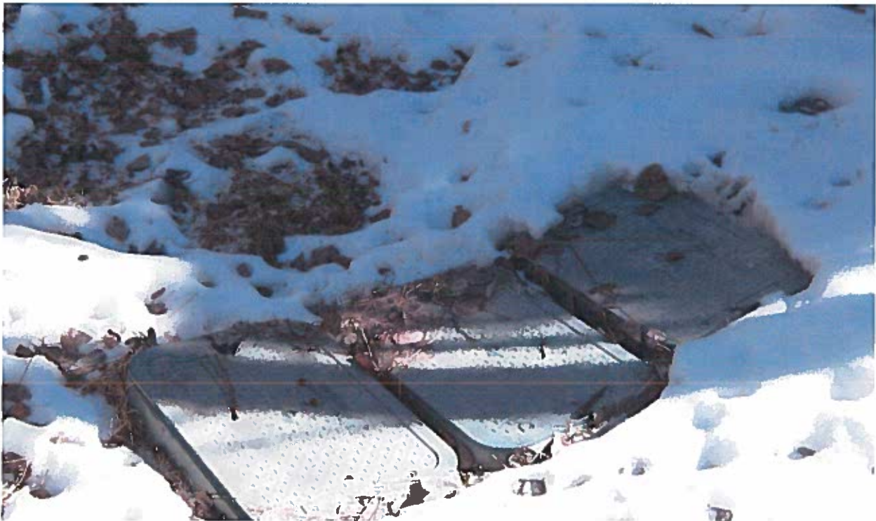
Irrigation system control boxes
