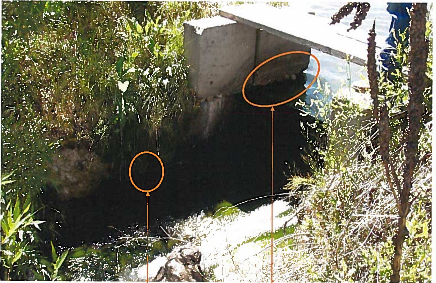
Above: Primary spillway: est 20 gpm leak discharging from right side. Suspected infiltration point at concrete joint.
