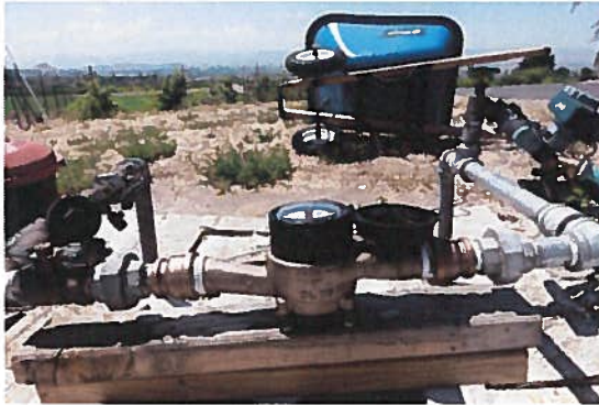
Water Meter In Gallons
