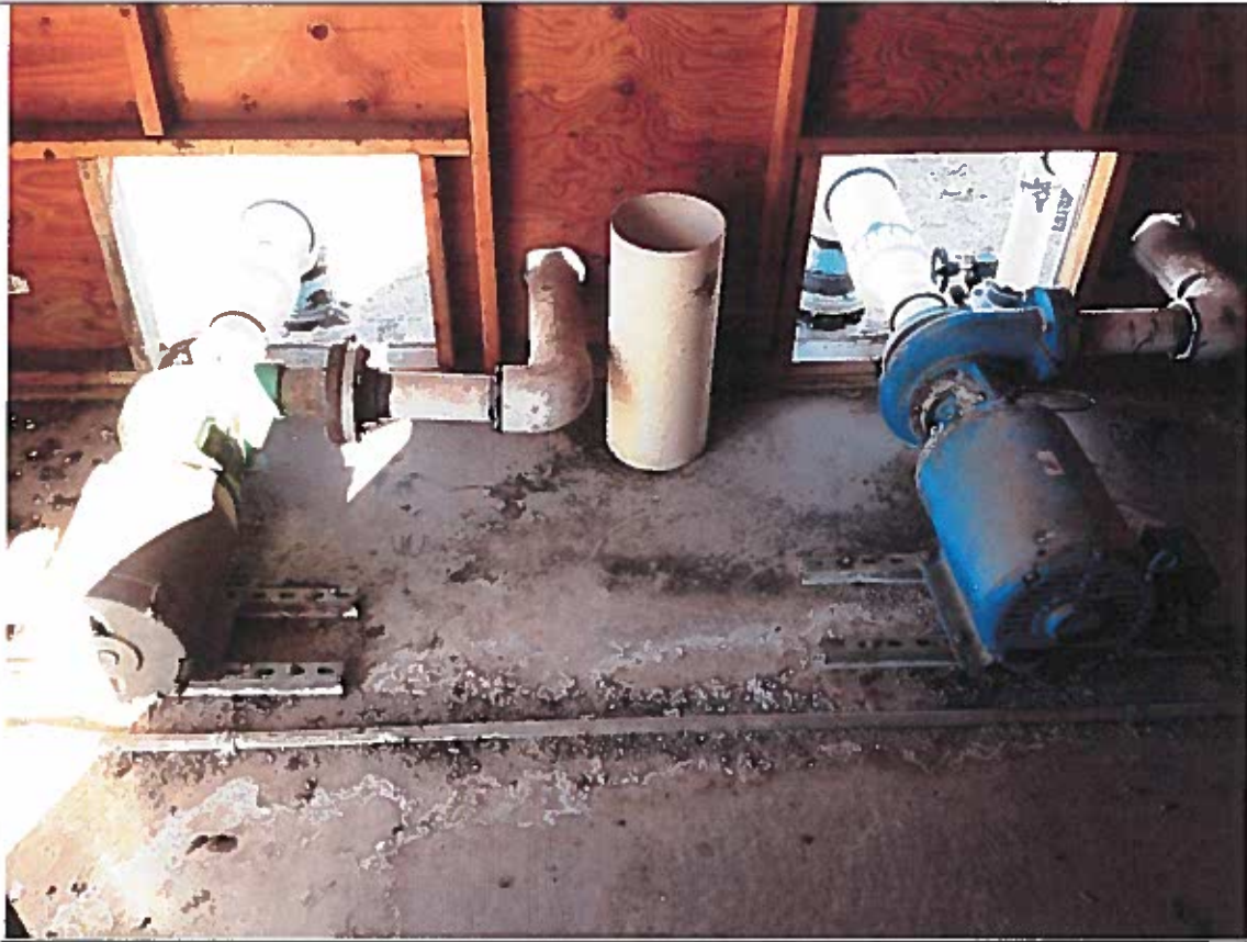
Two booster pumps stationed inside sprinkler pump house.
