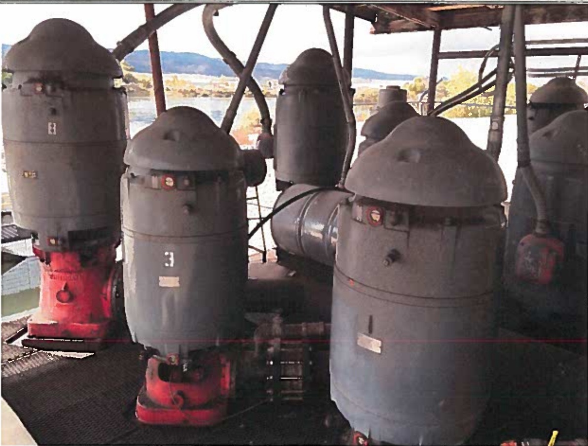
Pumps are lined in three rows of three, 9 pumps total, labeled as shown. (There is no No. 7)
