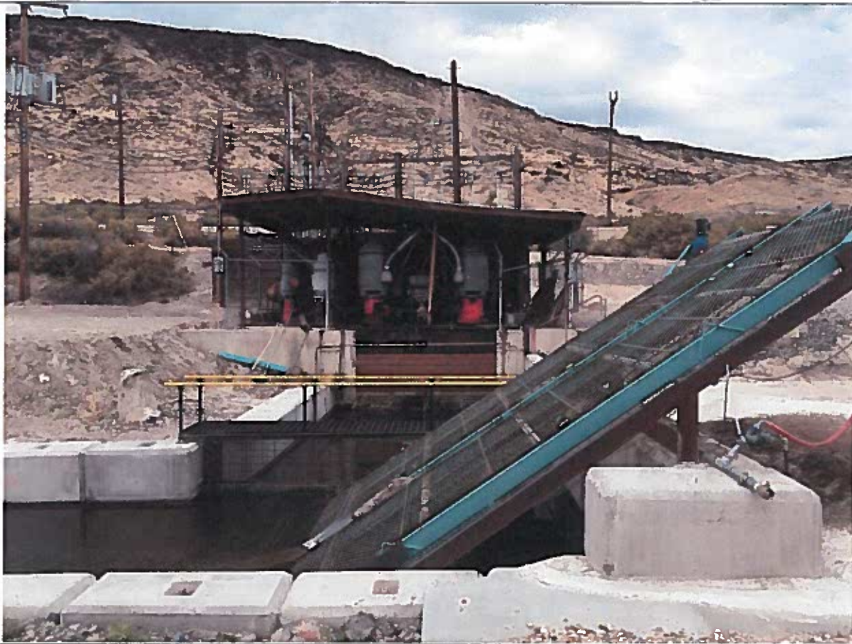
Pumping station looking north. Water is delivered above ridge in photo.
