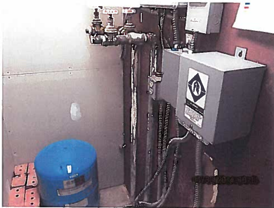
Pump room. Manual switch to storage.
